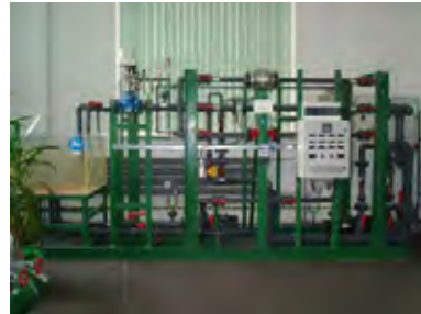
Hands-on facility of Pump
