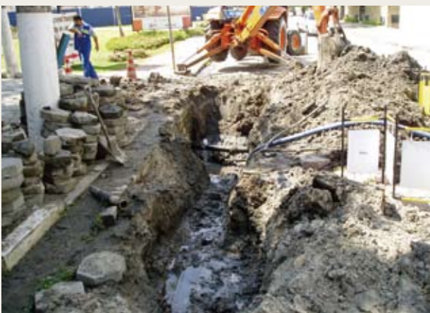
Water leak and repair
