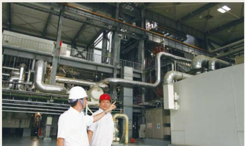
A new cogeneration facility. With consideration given to minimizing noise in the surrounding areas, the facility's gas turbine has been enclosed inside a large case (far right).
