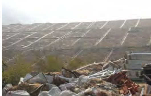
Fig. 9 Sub-project 4-2) Garbage Sanitary Filling Yard Construction Project in Changsha City: Filling yard side ditch
