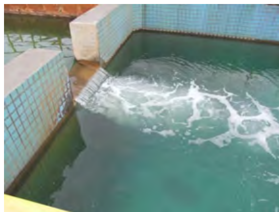
Fig. 5 Sub-project 2-2) Wastewater Treatment Project for Zhuzhou Chemical Factory: Treated water is of quality fit for direct discharge to Xiang River.
