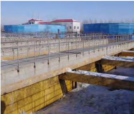
Fig. 2 1-3. Daqing Wastewater Treatment Plant
