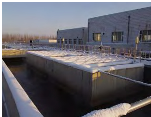
Fig.3 West suburb sewage treatment plant in Changchun City
