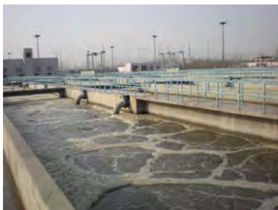
Fig. 2 Reaction Tank in a Sewage Treatment Facility in Zhengzhou
