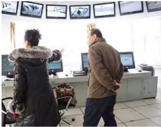
Fig.11 Central control room of Songyuan sewage treatment plant
