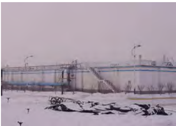
Fig.2 Sewage treatment plant in Songyuan City
