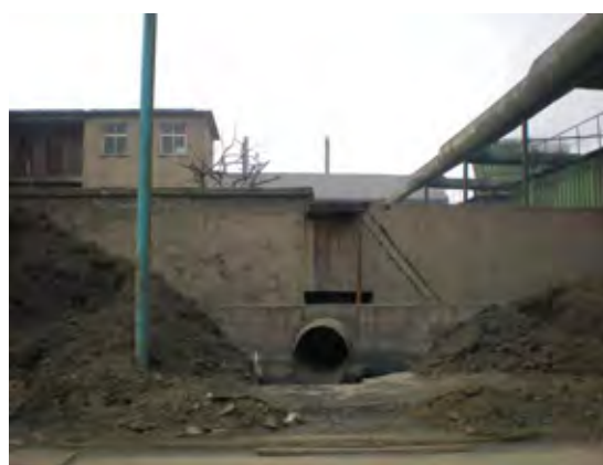
Fig.3 After Equipment Removal, Kaifeng Chemical Fertilizer Plant Waste Water Synthetic Treatment Project
