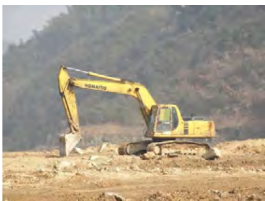
Fig. 8 Sub-project 4-2) Garbage Sanitary Filling Yard Construction Project in Changsha City: Equipment (a backhoe excavator)
