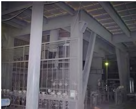
Fig. 4 3-2 Heat Supply Equipment in Yichun
