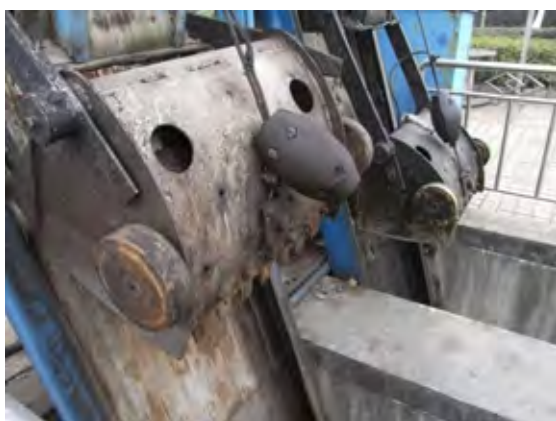
Fig. 2 Sub-project 1-6) Sewage Treatment Project in Xingsha Development Area of Changsha: wide-mesh screen
