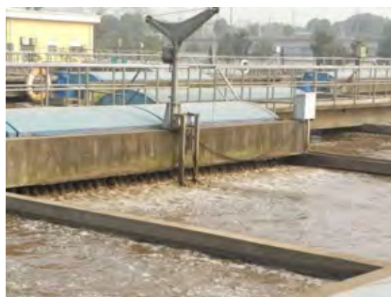
Fig. 3 Sub-project 1-8) Expansion Project of Changsha No.1 Sewage Treatment Plant: oxidation ditch process-based treatment facility
