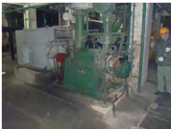
Figure 1.3-20 Boiler feed pump
