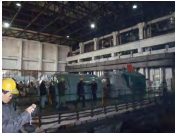
Figure 1.2-1 Turbine and generator
