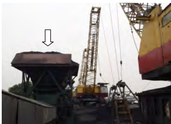
Figure 1.3-4 Belt conveyor hopper for the coal acceptance (indicated by an arrow)
