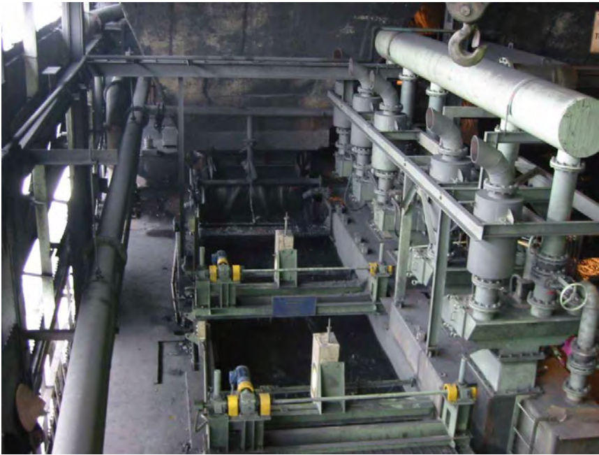
Figure 3.3-4 JIG (Cua Ong preparation plant)
