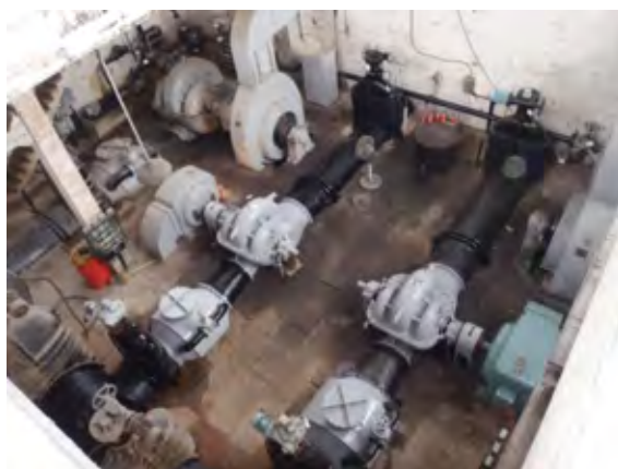
Figure 1.3-19 Circulating water pump
