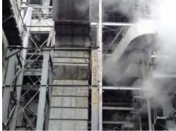
Figure 2.2-7 Status of duct
