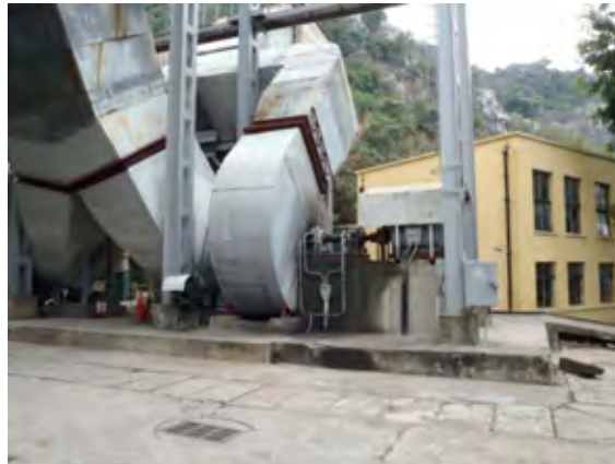
Figure 1.3-15 Induced draft fan
