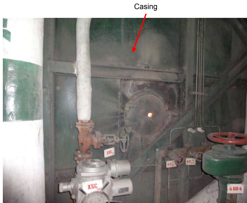
Figure 2.2-4 Status of boiler skin casing
