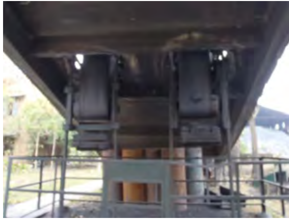
Figure 1.3-7 Conveyor-belt tensional adjuster
