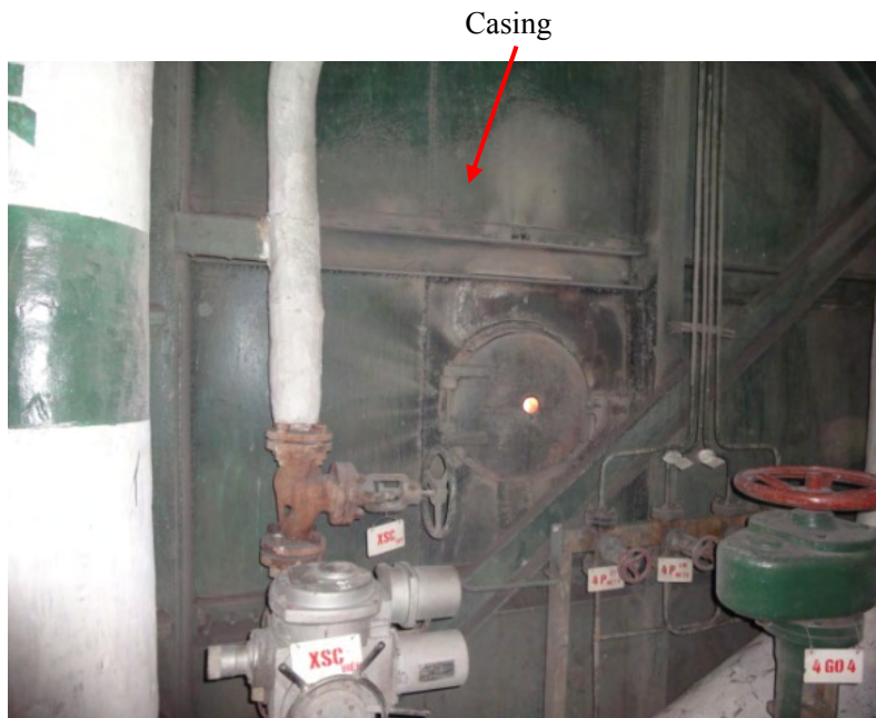
图 2.2-4 Status of boiler skin casing
