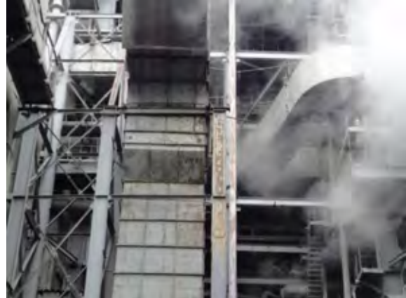
図 2.2-7 Status of duct
