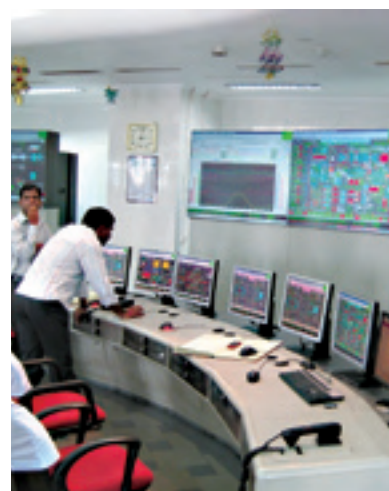
Central Control Room
