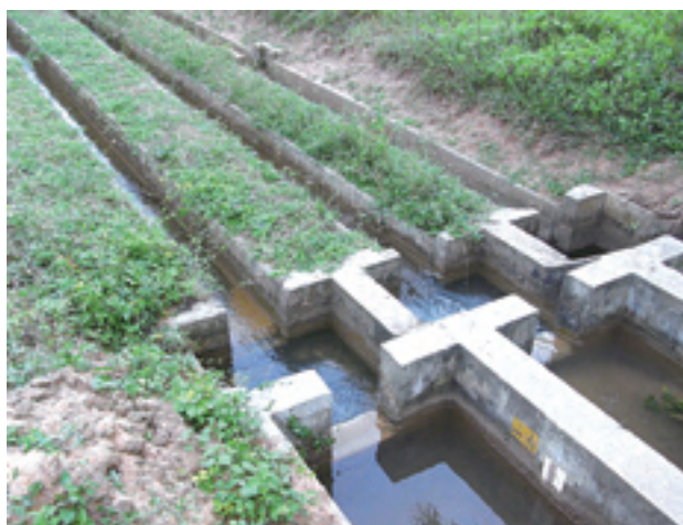
A canal constructed by the Walawe Left Bank Irrigation Upgrading and Extension Project
