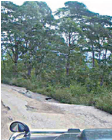
A road with surface damage
