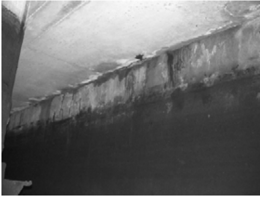
Wall nearby Pile 25C
