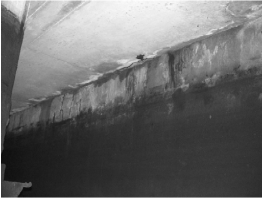
Wall nearby Pile 25C
