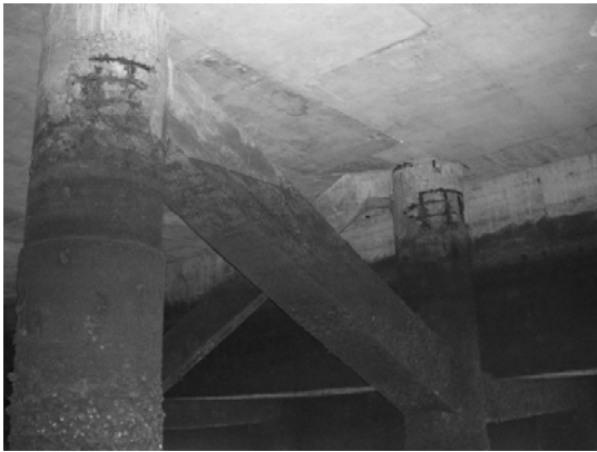
Block 3 Brace bet. Pile 43F & 43G
