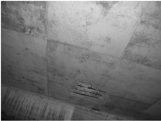
Block 2 Slab bet. Pile 20A & 21A
