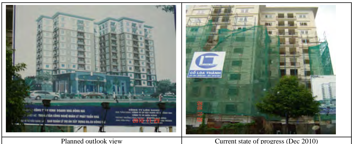
Figure 11.4.5 Pictures of Resettlement Building at Nguyen Van Troi Str., Quang Vinh Ward
