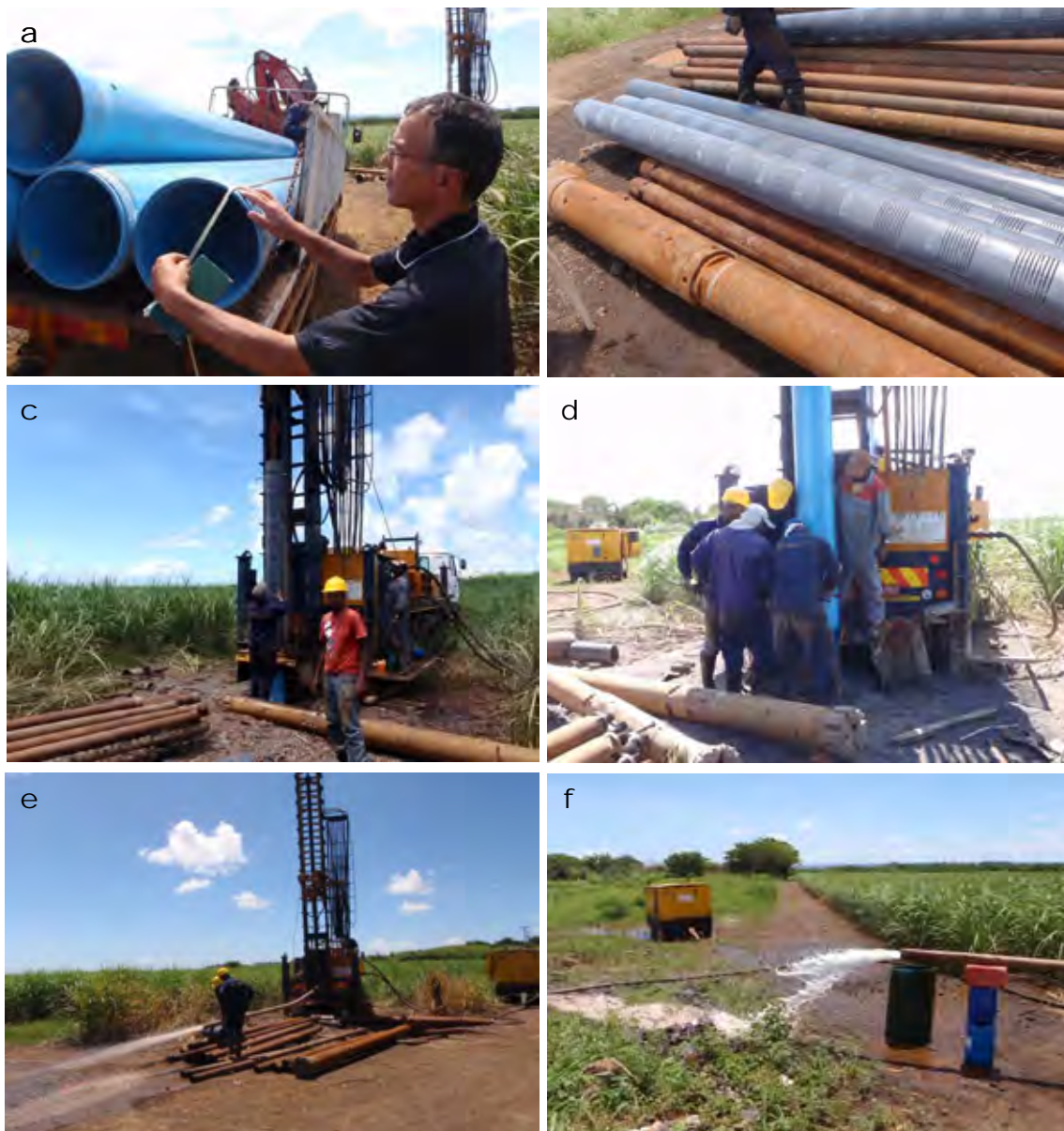
Figure 4.3-3 (a) Casing of PVC Pipe with 300 mm Diameter; (b) Slotted PVC Pipes; (c) Installing the Casing into the Borehole; (d) Installed Casing with Blue Filter; (e) Cleaning by Airlift; (f) Discharge of Airlift
