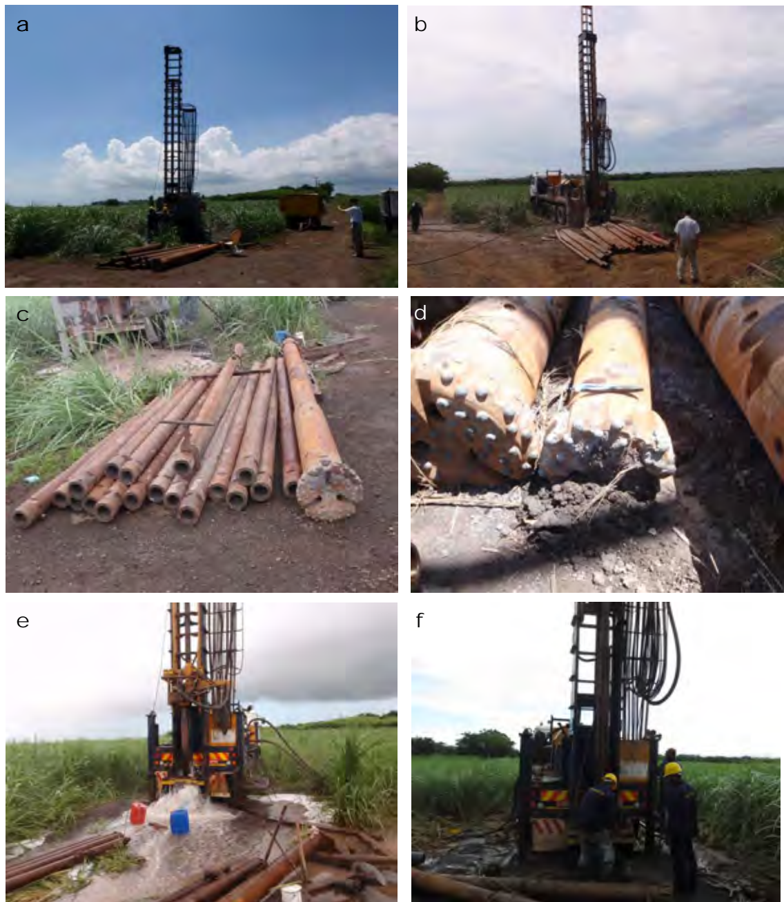
Figure 4.3-2 (a) Drilling of BH-4 by Down-the-hole Hammer; (b) Drilling of BH-5 by Down-the-hole Hammer; (c) Down-the-hole Hammer Bit and Rods; (d) Bit with diameter of 300 mm; (e) Drilling with water at BH-4; and (f) Drilling at BH-5
