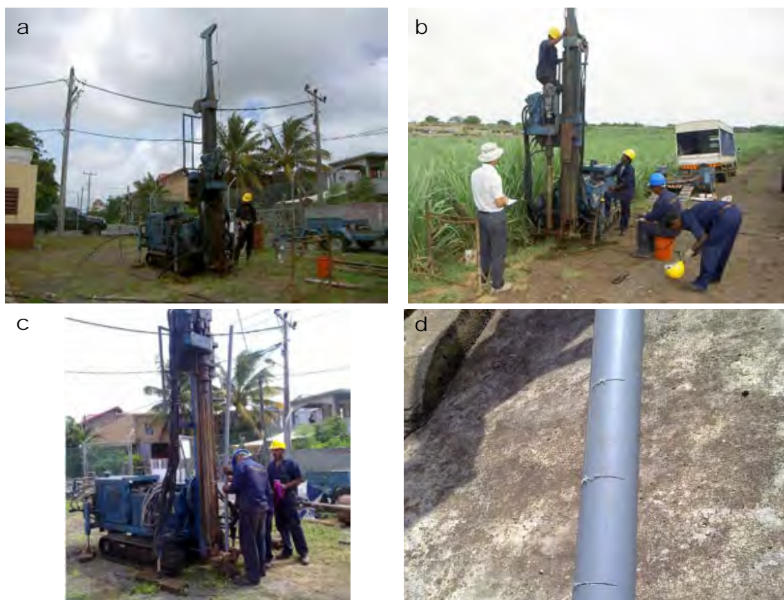
Figure 4.2-2 (a) Drilling the Core Hole by Rotary Boring Machine; (b) Conducting SPT; (c) Installation of Standpipes for Groundwater Level Gauge; and (d) Slotted Tube for Standpipes.
