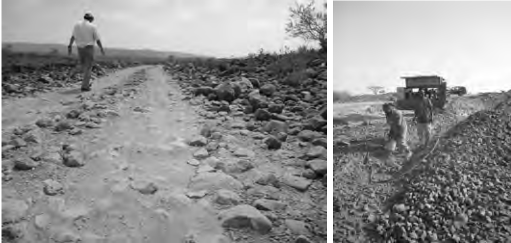
Figure 2-2-24 Generally, Construction Site is covered by Basalt (hard rock) (Left Figure) Breaker is used to Excavate Basalt Ground (Right Figure)
