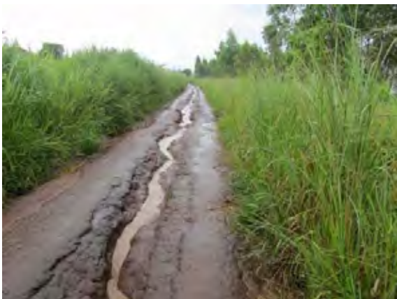
Before the Project (Eroded due to lack of side drain)
