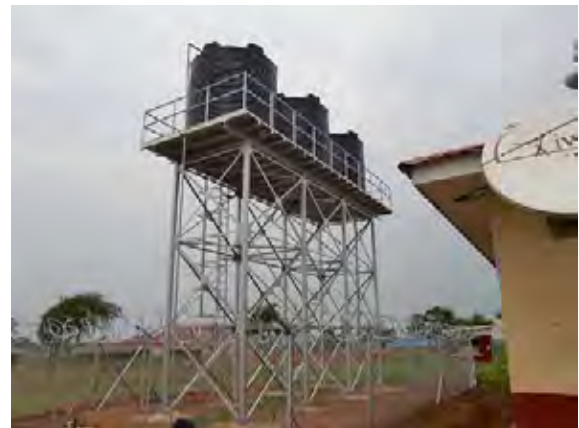
Water Storage facility (30,000lt water tank)
