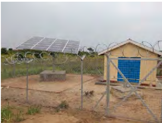
Installed Solar Panel and Pump House
