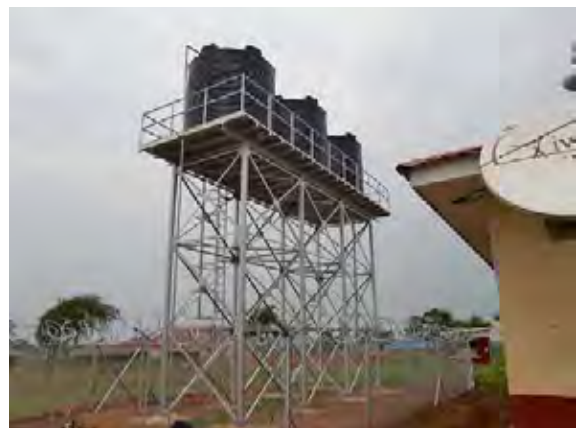
Water Storage facility (30,000lt water tank)
