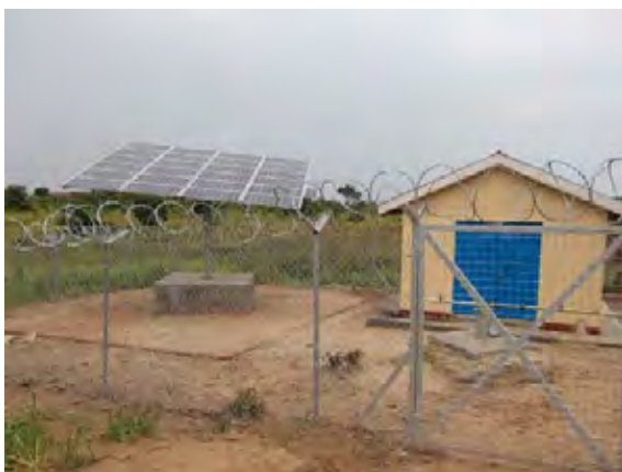
Installed Solar Panel and Pump House
