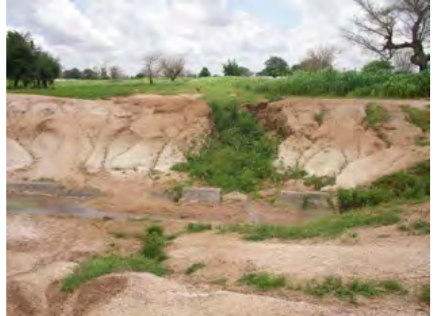
Right Main Canal : Excavated Section Deteriorated section by drainage water from outside
