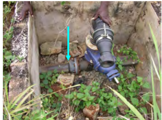
Leakage joint portion (pointed by an blue arrow)
