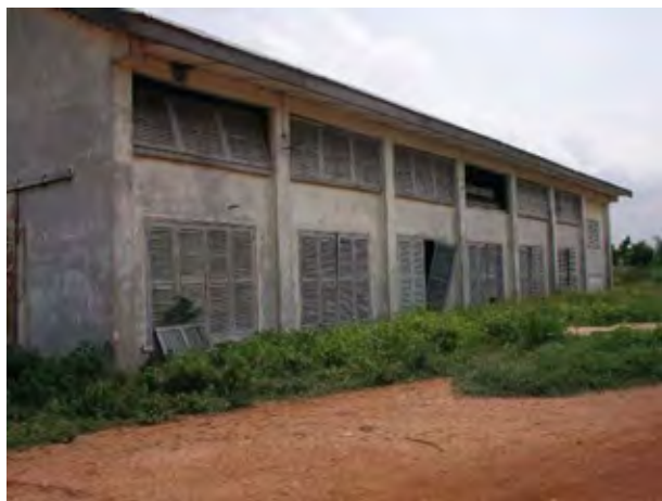
Pump station is not in use because of deterioration.
