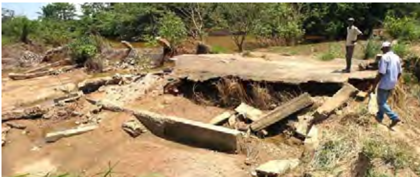
Damaged part by Flood at the intake site Protection Dyke and Spill way were washed out
