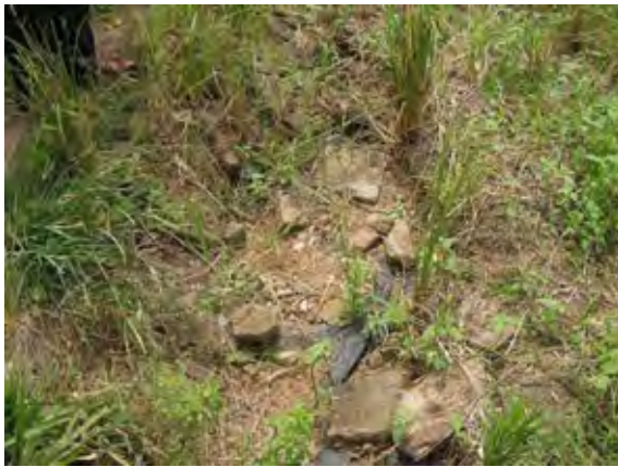
Deteriorated secondary canal. Trace of block lining was seen.
