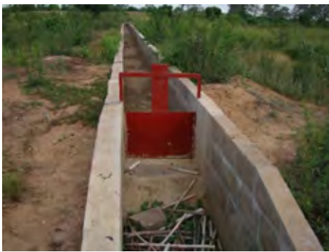
Cross Regulator: Canal wall on left side is thick because of restoration works after falling down.
