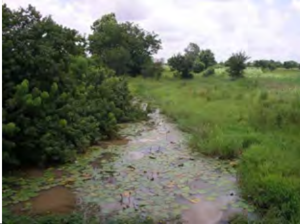
Main Drainage Canal : Canal flow section is almost closed by grasses and sedimentation.
