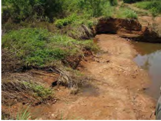
Broken dyke near the pump station
