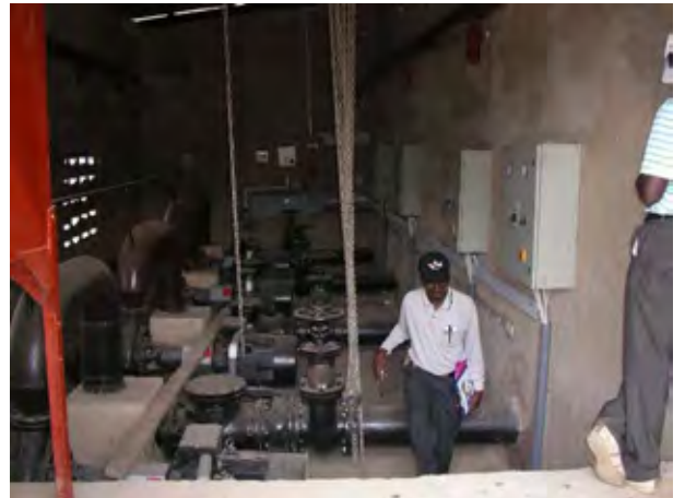
Four pump units are installed.
