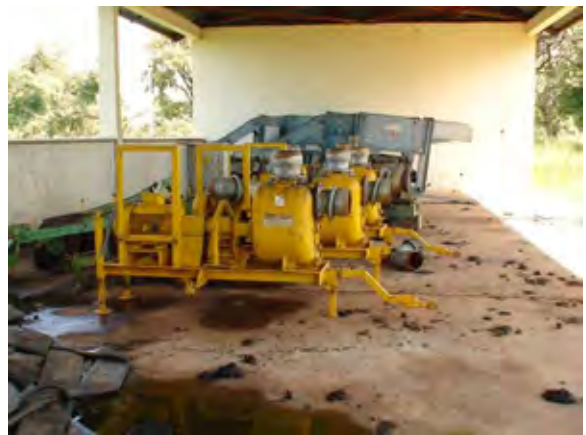
Pump rusting from lack of use
