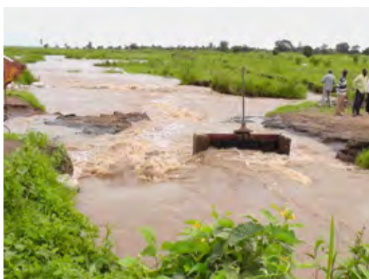
Main canal diversion works downstream have been swept away
