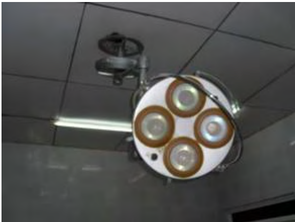
Tbat Rural Hospital (Gezira), Operation room The lamp has no bulbs and is hung in midair.
