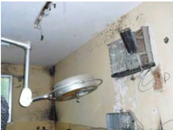
Singa Teaching Hospital (Sinnar), Operation room The electric wirings are exposed.
