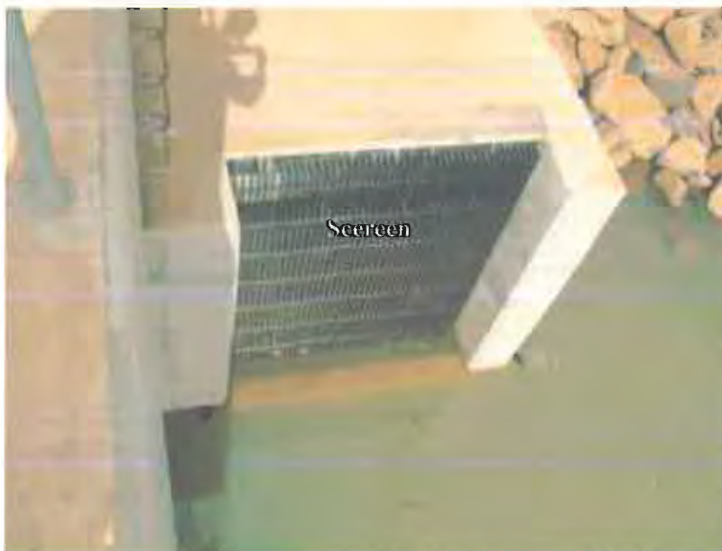
Intake of O'Moleg Power Station
