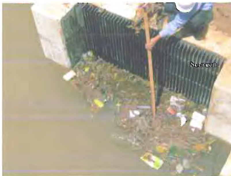
Status of debris on screen of O'Moleng Power Station
