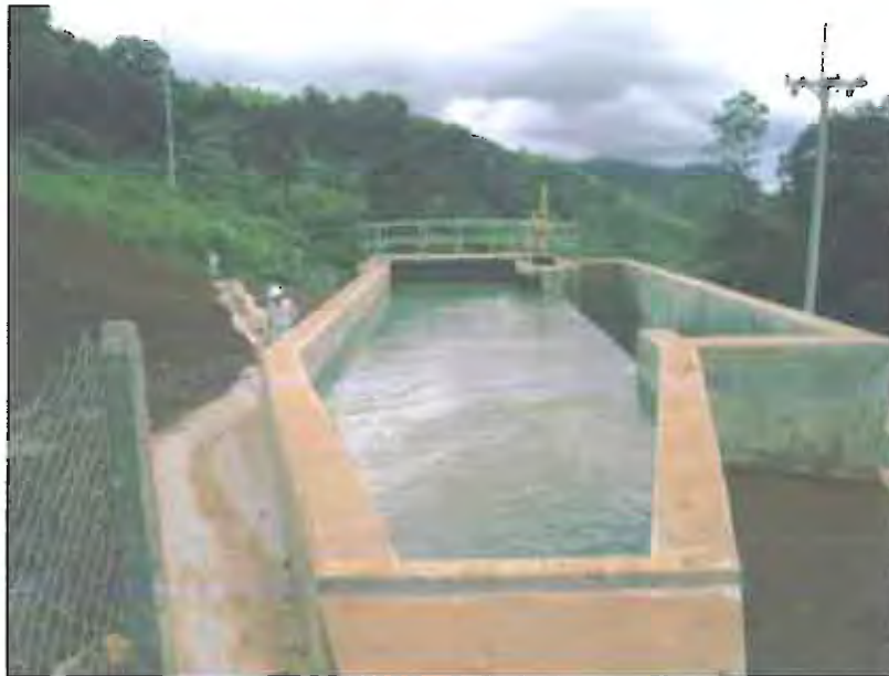
Head tank of O'Romis Power Station
