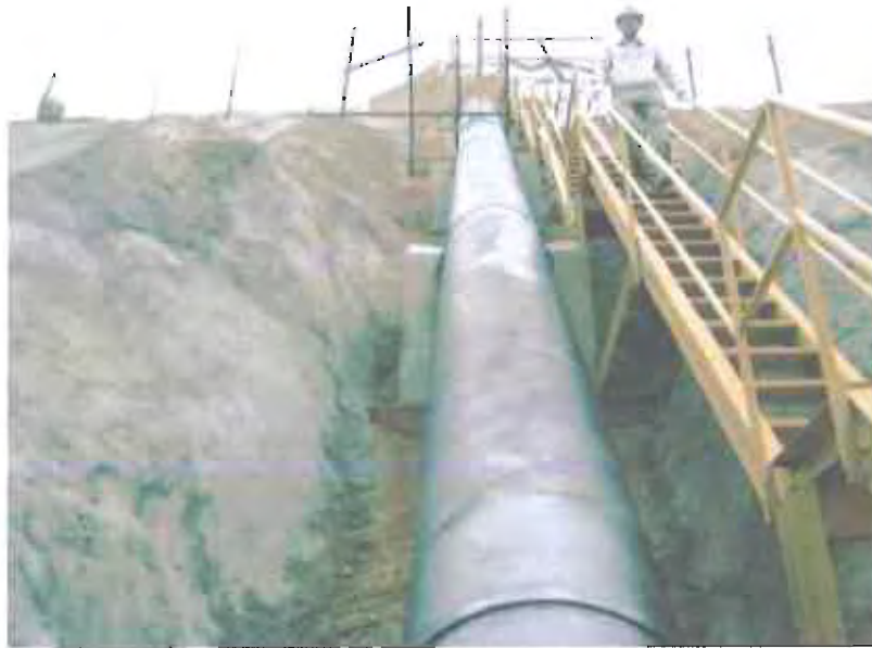
Penstock of O’Romis Power Station
