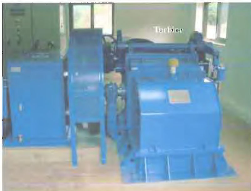
Turbine generator of O'Moleng Power Station
