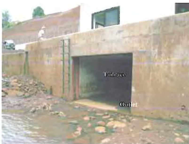
Tailrace of O'Romis Power Station
