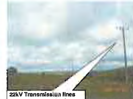
22kV Transmission Lines
