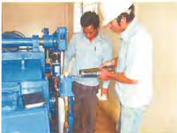
Grease up for turbine bearings
