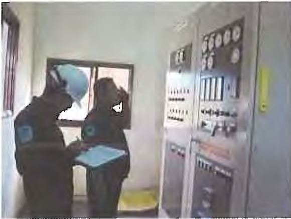
Trial Operation after Inspection
