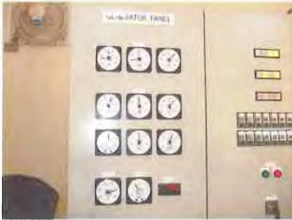
Trial Operation after Inspection
