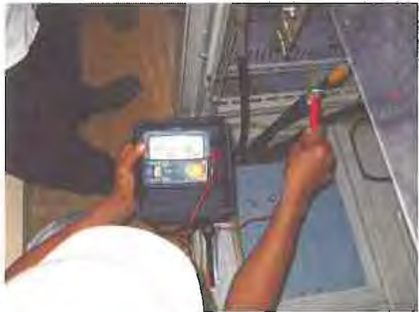
Measuring Insulation resistance of Generator
