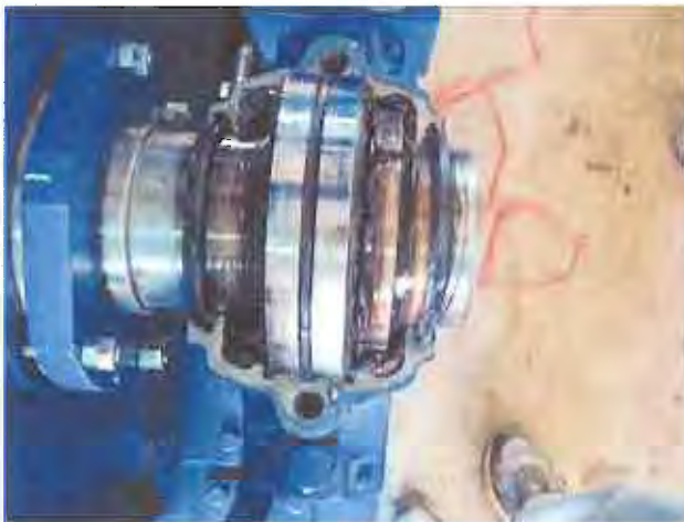
3. Grease change for turbine bearings
