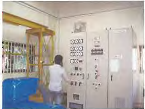
8. Trial operation after inspection
