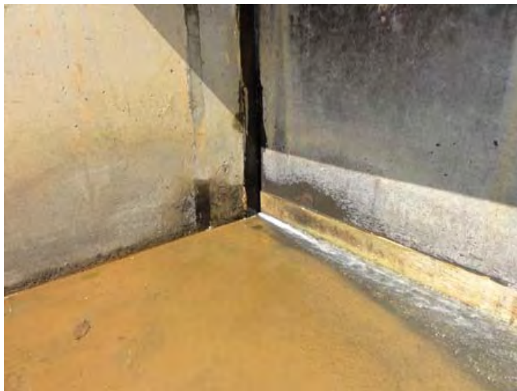
○ Guidance in patrolling (O'Moleng Power Station) Leakage from the sand removal gate
