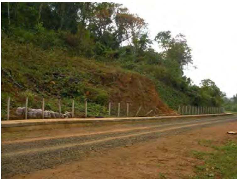
[For reference] State of the slope before the repair (December 2009)
