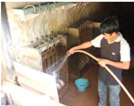
Inspection and Cleaning of Dummy Load at O'Moleng P.S
