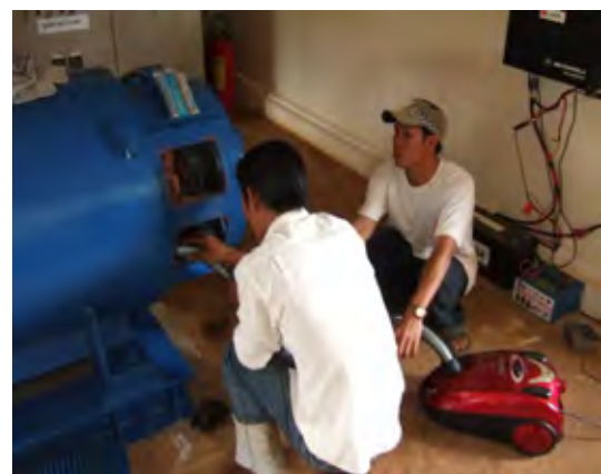
Generator inspection and cleaning at O'Romis P.S
