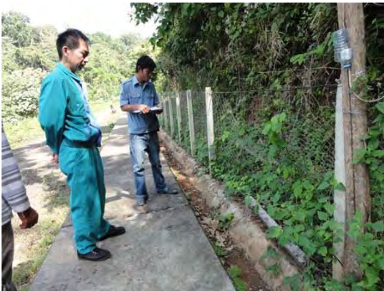
○ Patrol in progress (O’Romis Power Station) Fallen posts of rockfall protection fence
