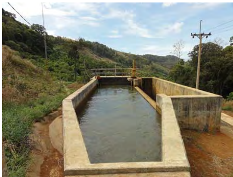
○ O'Romis Power Station Present state of water tank. There was no overflow into the effluent outlet. Hydropower when photograph taken: 140 kW.
