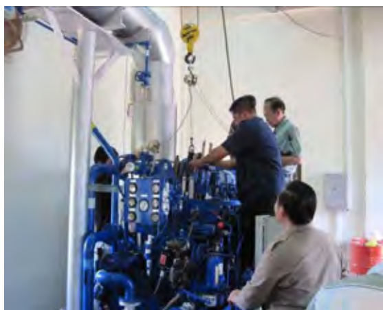
DG disassembly inspection 4,000—5,000 hours
