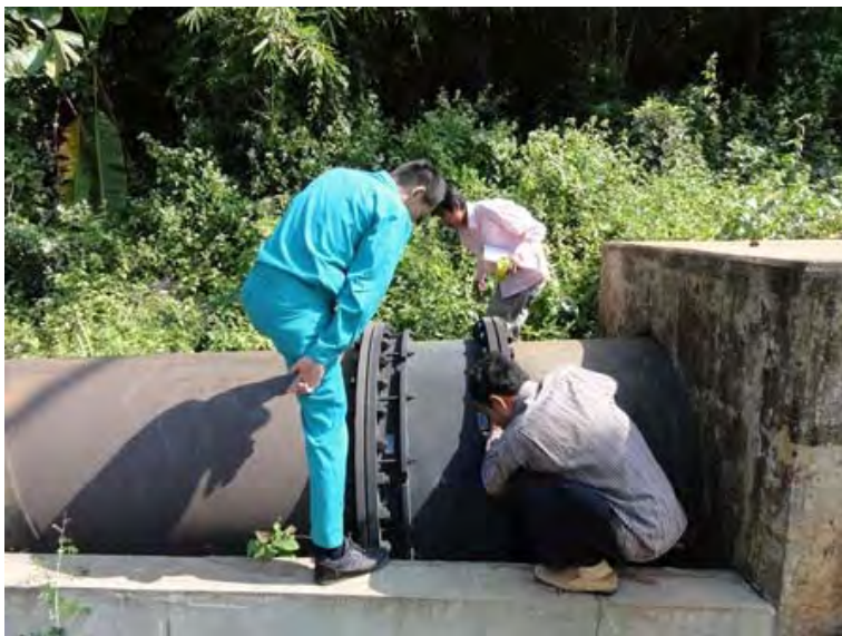
○ Patrol in progress (O'Moleng Power Station) Inspecting a joint portion of the hydraulic pressure iron pipe
