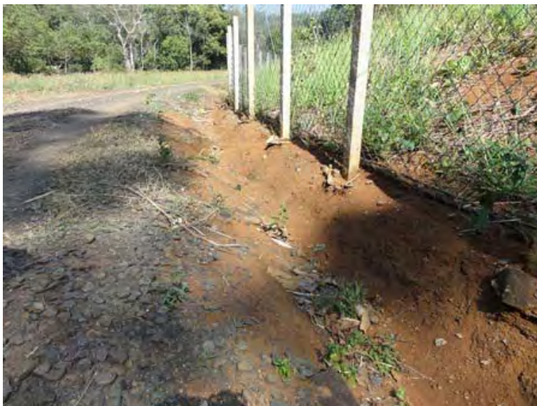
○ Guidance in patrolling (O'Moleng Power Station) Base portions of posts in rockfall protection fence along access path
