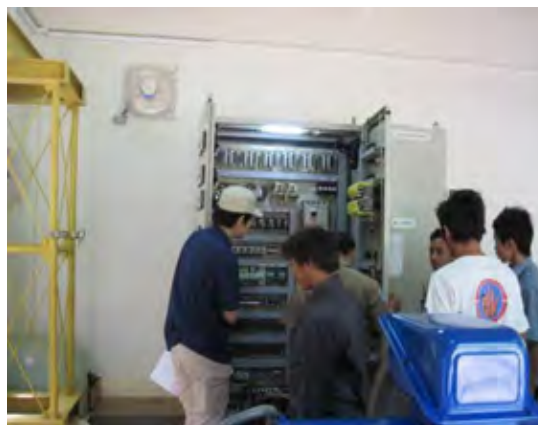
Inspection and Cleaning of Control Panel at O'Moleng P.S
