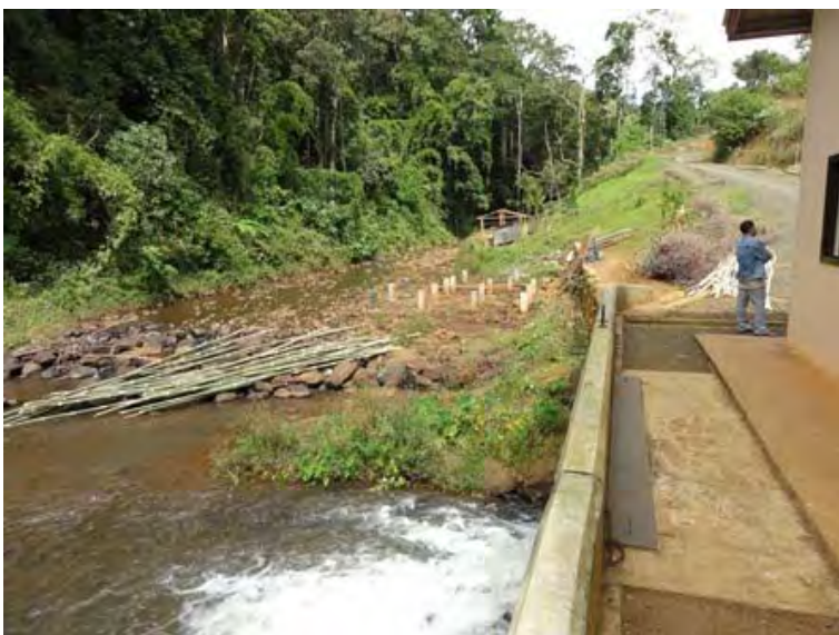
○ O'Romis Power Station Dwelling that had been erected on the river had been removed (leaving only the foundations).
