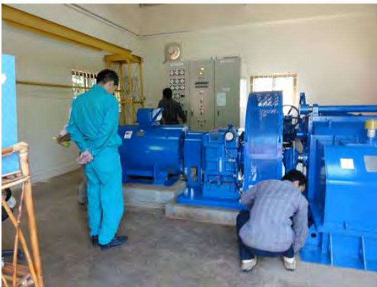
○ Patrol in progress (O'Moleng Power Station) Inspecting the bases of machinery inside the building
