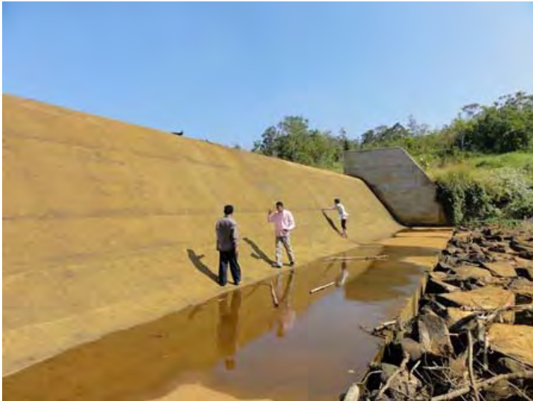
○ Guidance in patrolling (O'Moleng Power Station) Seepage at the diversion weir joint portion.
