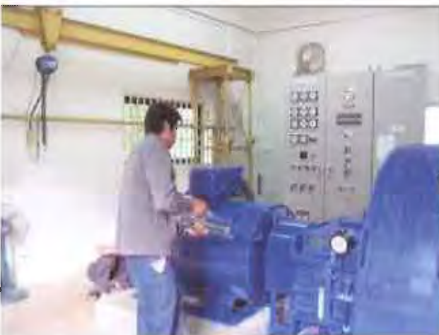
Grease up into generator bearings
