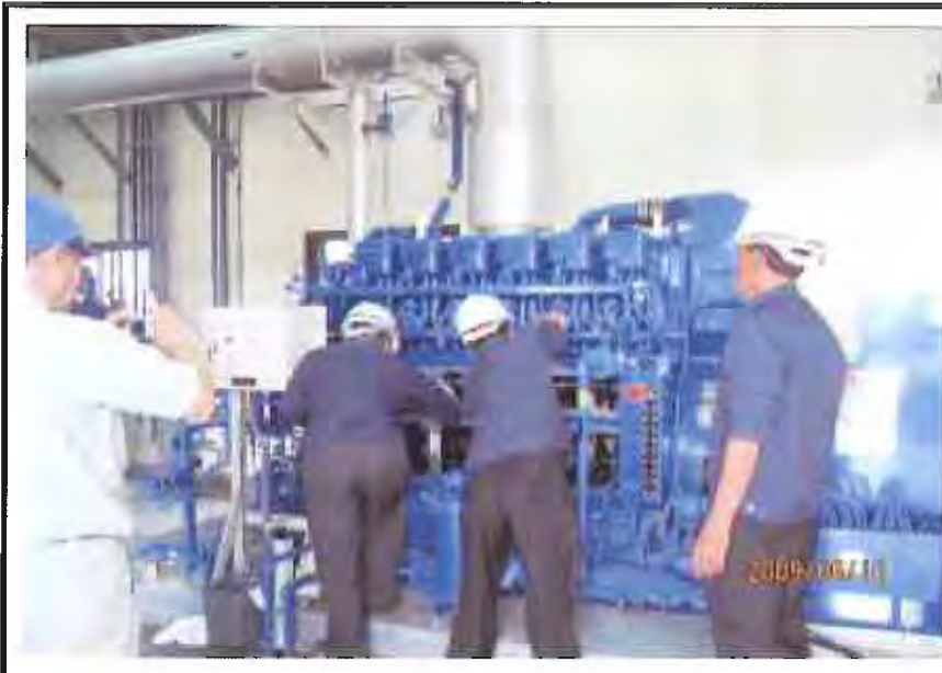
Periodic Inspection and OJT for Diesel engine (Disassembly of Engine body)
