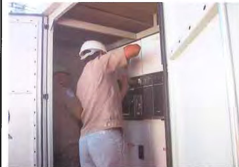
Operation of Switchgear at Scheduled Outage
