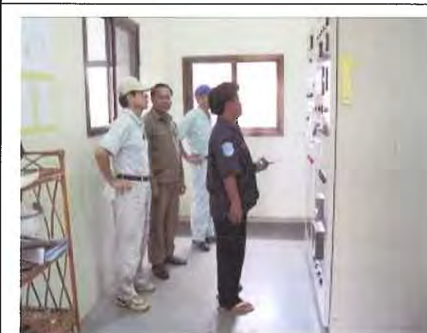
Trial Operation after Periodic Inspection
