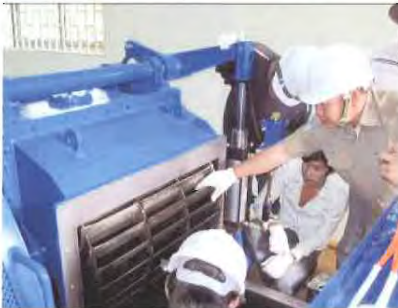
Periodic Inspection and OJT for Turbine inside Runner at O'Moleng Hydropower Station
