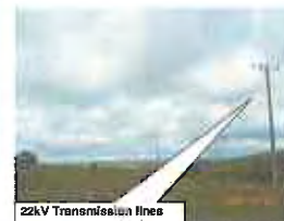
22kV Transmission Lines
