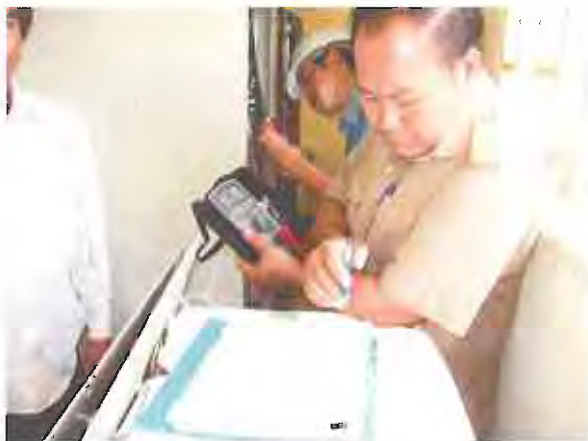
Measuring Insulation resistance of dummy load
