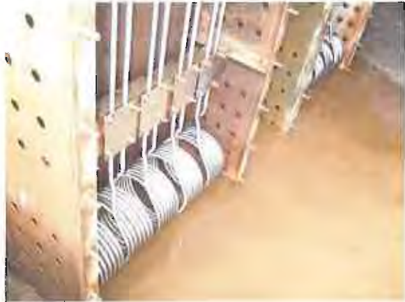
Cleaning of Dummy load
