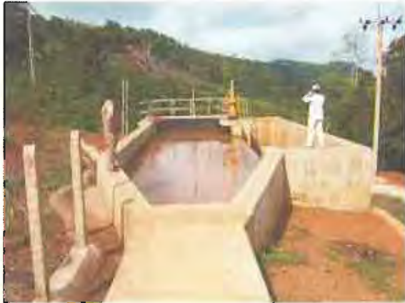
Drought condition at O'Romis Hydropower station (Head Tank)
