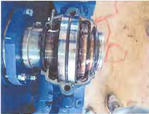
3. Grease change for turbine bearings
