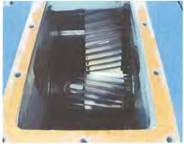
6. Inspection inside of speed gear
