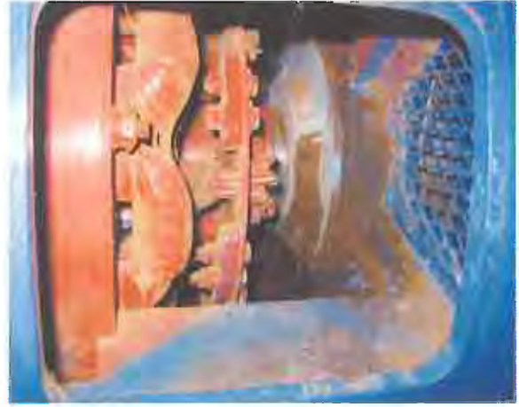
8. Inside of generator (dirty condition)
