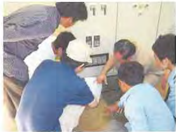
OJT for protection relays and manual on the control panel at O'Moleng.
