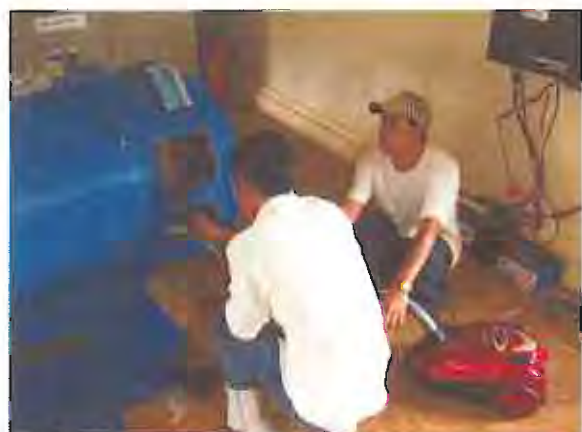
Inside inspection and cleaning of generator
