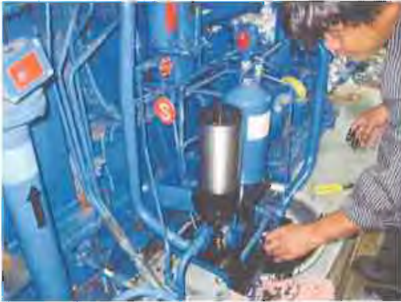
Cleaning of Engine Lubricating oil filter
