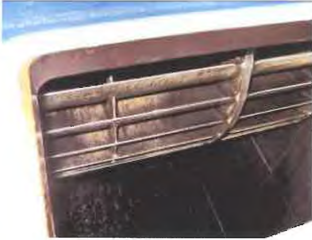
Turbine runner inside
