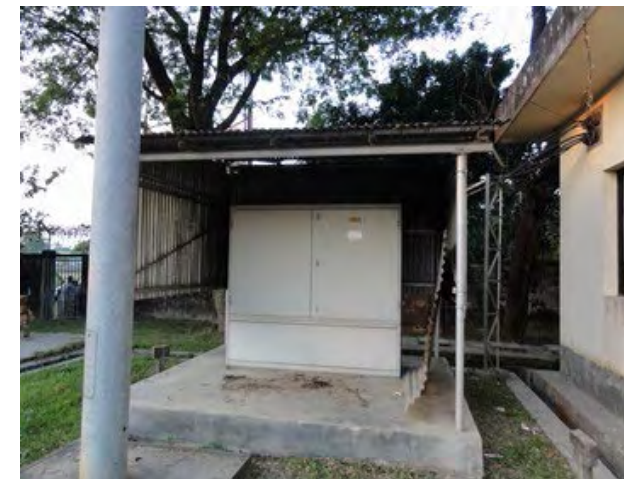
Existing RTU (cable link)
