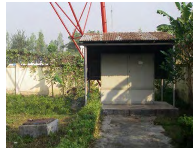
Existing RTU (cable link)
