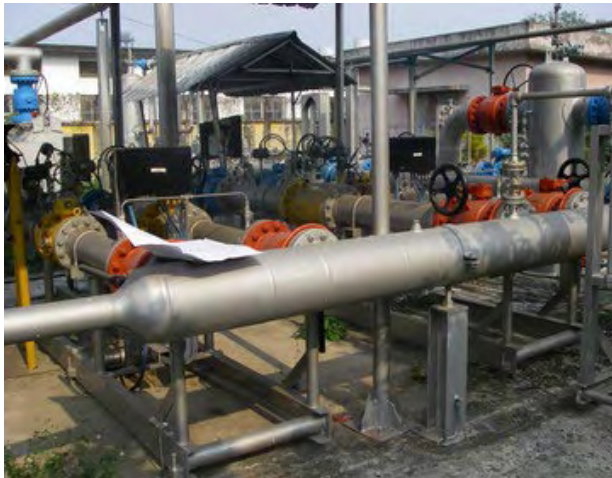
New gas pipelines to be monitored
