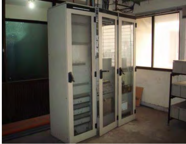
Existing Radio Equipment Room located at 9F of commercial building
