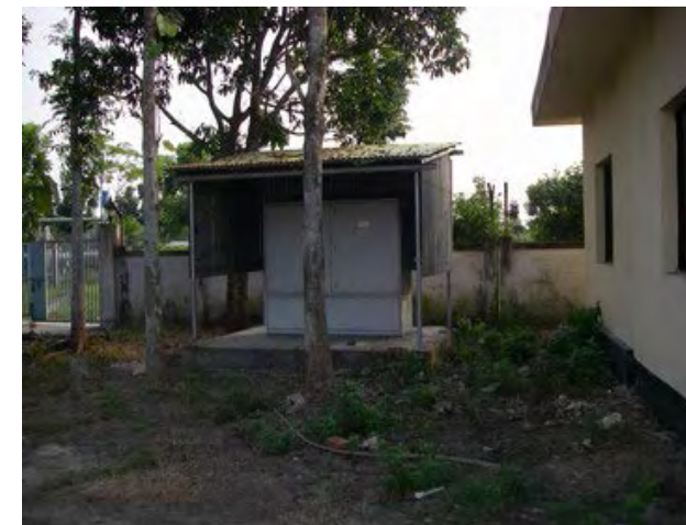
Existing RTU (cable link)
