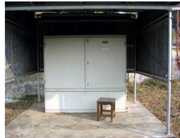
Existing RTU (cable link)
