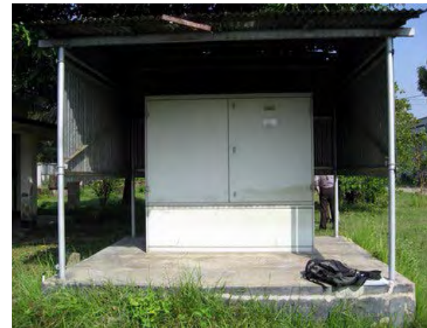
Existing RTU (cable link)
