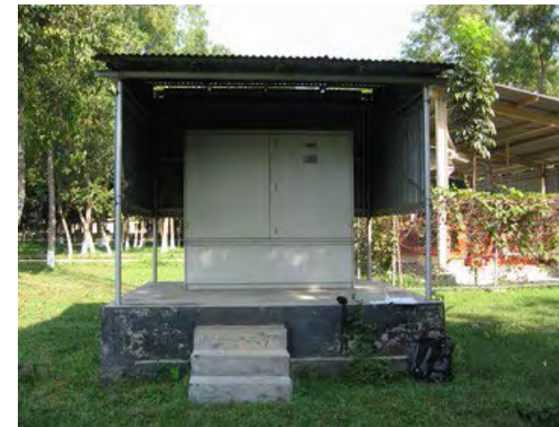
Existing RTU (cable link)
