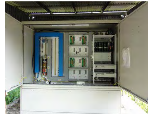
Existing RTU (cable linke)
