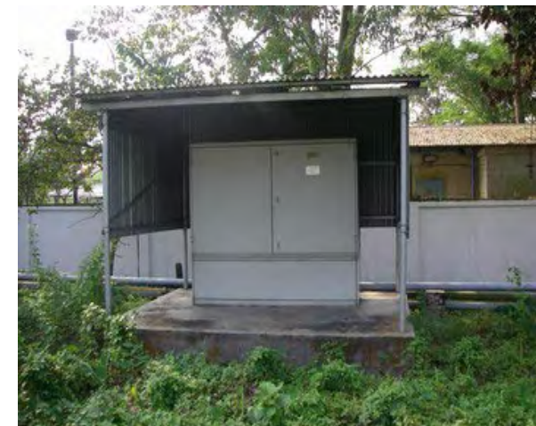
Existing RTU (cable link)
