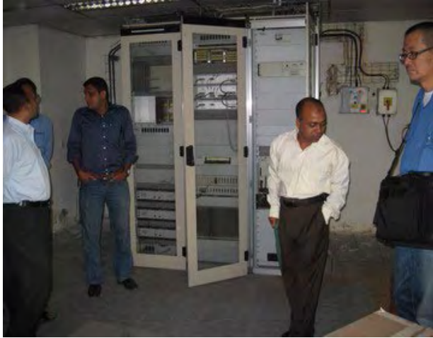
Existing Radio Equipment Room located at penthouse of commercial b
