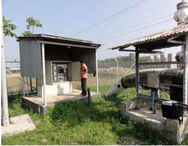
Existing RTU and Instrument Stand
