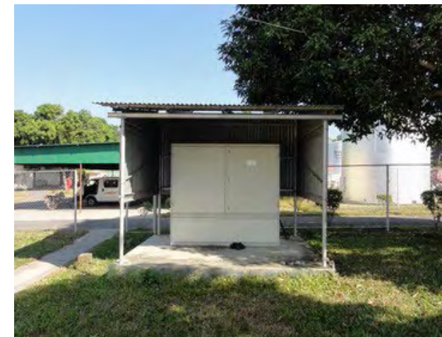
Existing RTU (cable link)
