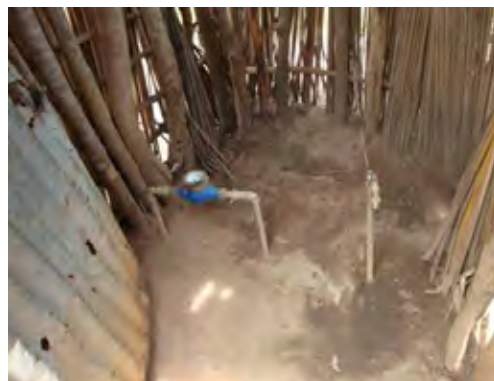
Yard Tap Connection
