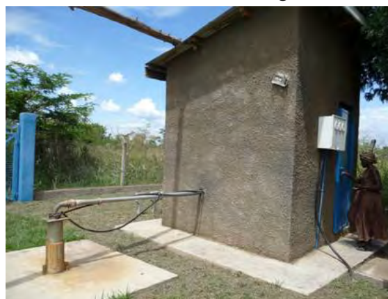
Intake Borehole for RGC
