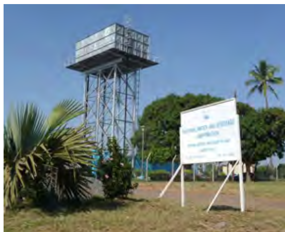
Photo 14-1 Water Tank (Soroti)
