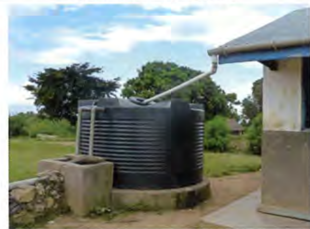
Rain water storage tank (Soroti District) [Nov. 2009]
