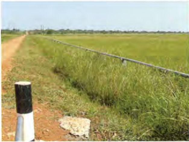
Transmission pipes to Soroti, Amuria and Kaberamaido (Soroti District) [June 2009]
