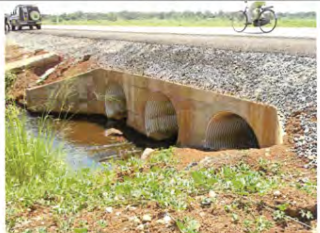
Simple bridge of trunk road. Sometimes being under water in rainy season. (Bugiri District) [June 2009]
