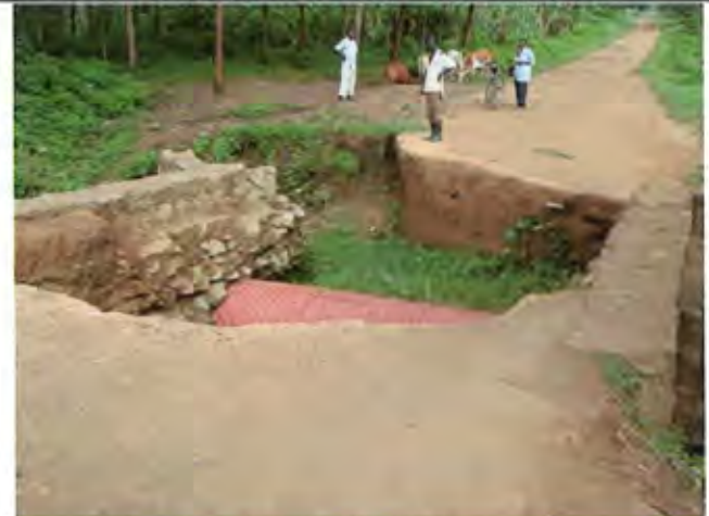
Exposed drainage pipe of simple bridge due to erosion in rainy season (Mbale District) [June 2009]
