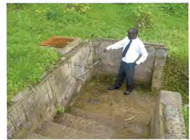
Intake facility of gravity scheme (Sironko District) [Nov. 2009]
