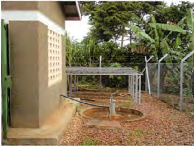
Solar powered water supply system (Nsozibili, Jinja District) [Aug. 2010]
