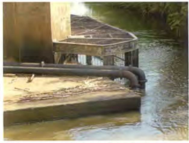
Intake Facility in Manafwa River for Mbale Municipality (Mble District) [July 2009]
