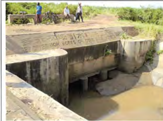
Intake facility of irrigation water supply system for Doho Rice Scheme blocked partially by Sedimentation. (Butaleja District) [Aug. 2010]
