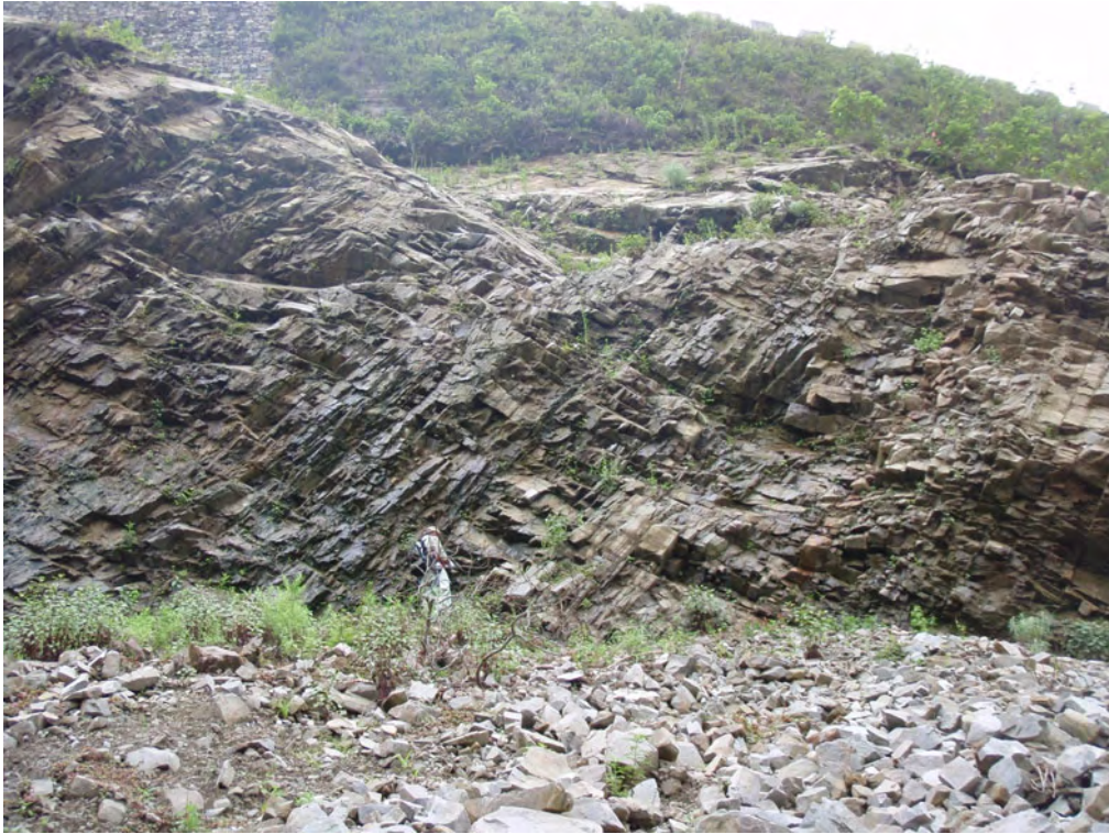
Photo.5 Cracked Quartz Schist at the upper part of the failure.
