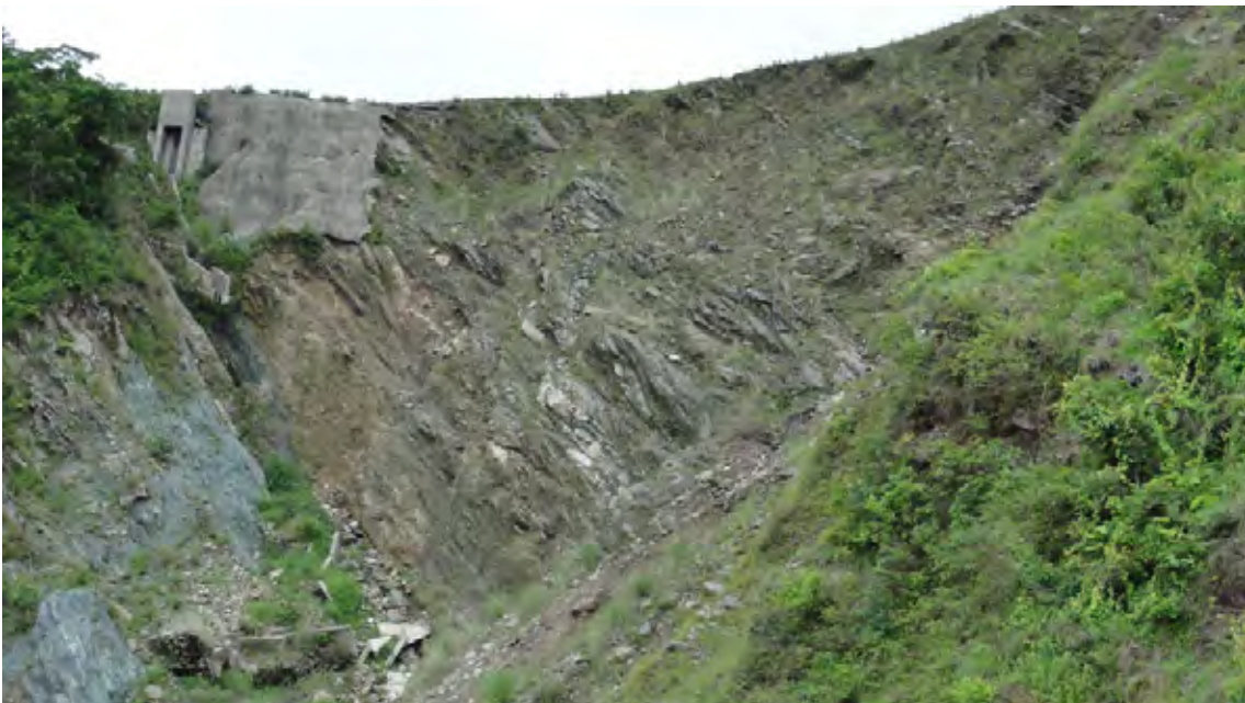
Photo.4 Failure at Sta.17+400.
