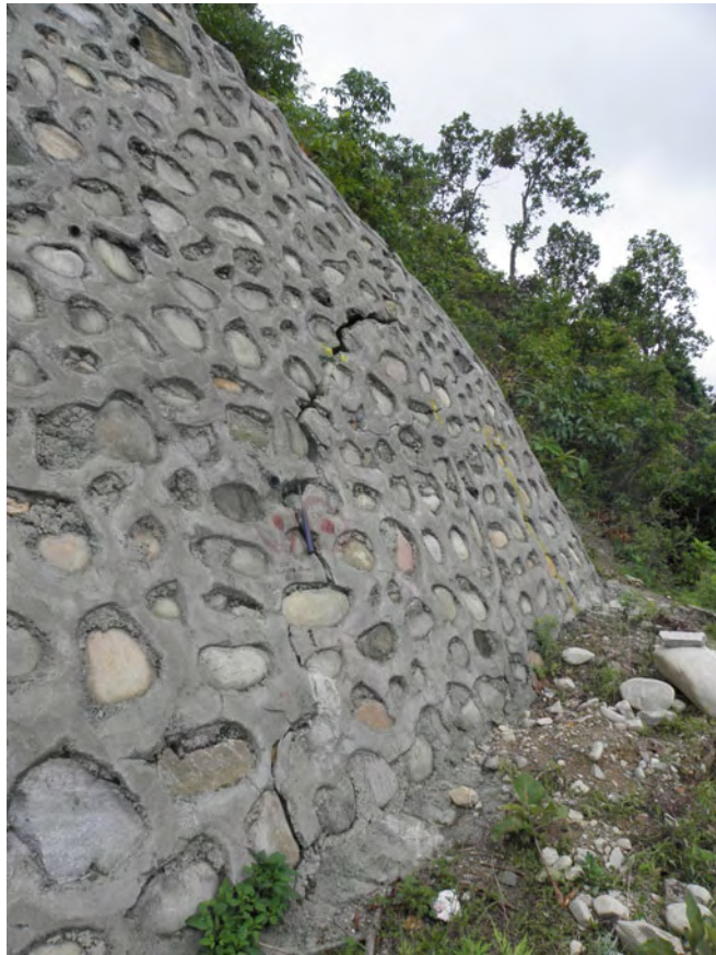
Photo.10 Cracks on the wall at Sta.18+200
