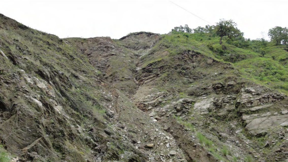
Photo.7 The lower of failure at Sta.18+200.
