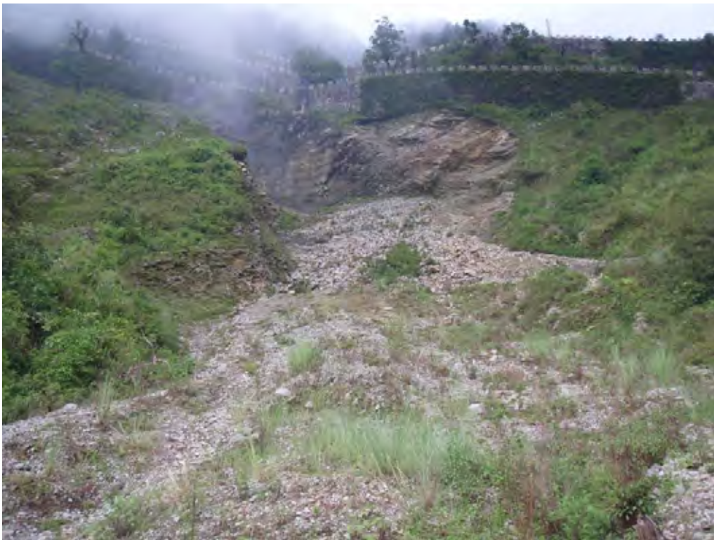
Photo.2 Full view of a failure at Sta.17+600 site. (from the lower of slope)
