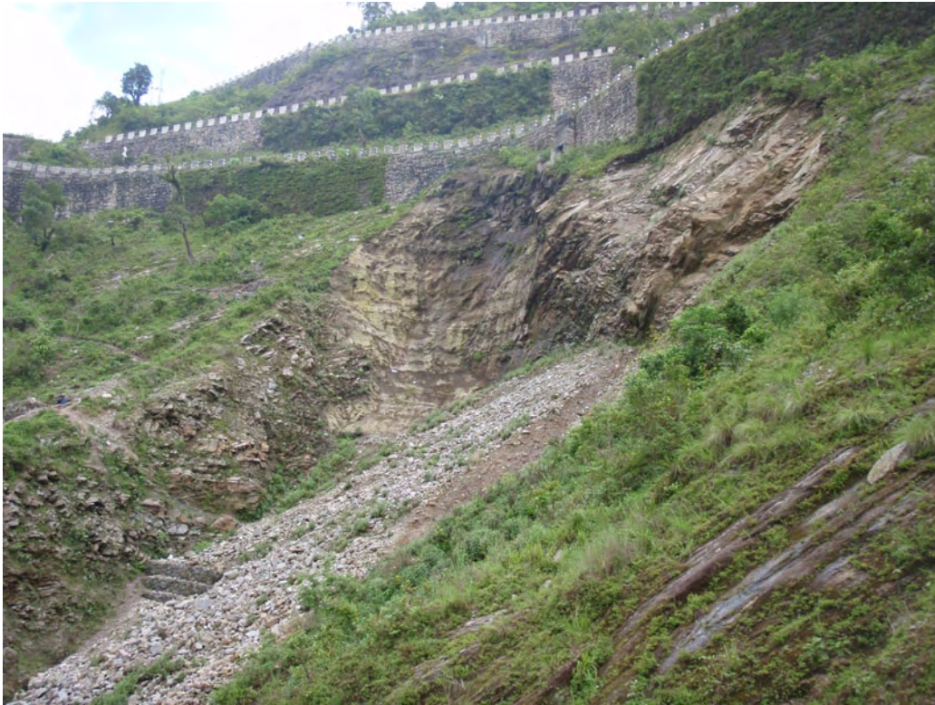
Photo.1 Full view of a failure at Sta.17+600 site.
