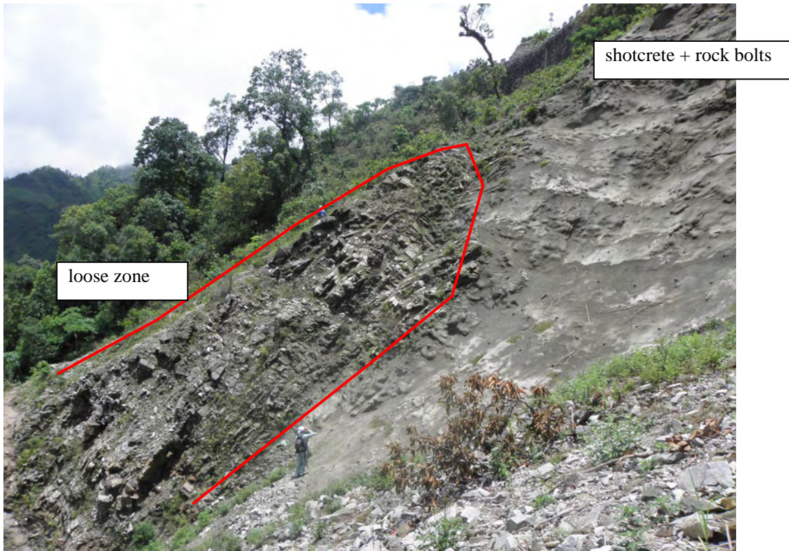
Photo.3 Loose zone under the failure at Sta.17+600.
