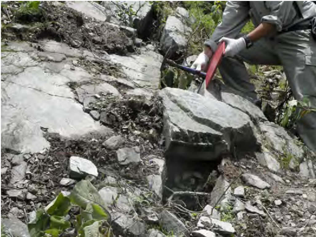
Photo.4 Crack on loose zone under the failure at Sta.17+600.(crack wide:43cm, N20W)
