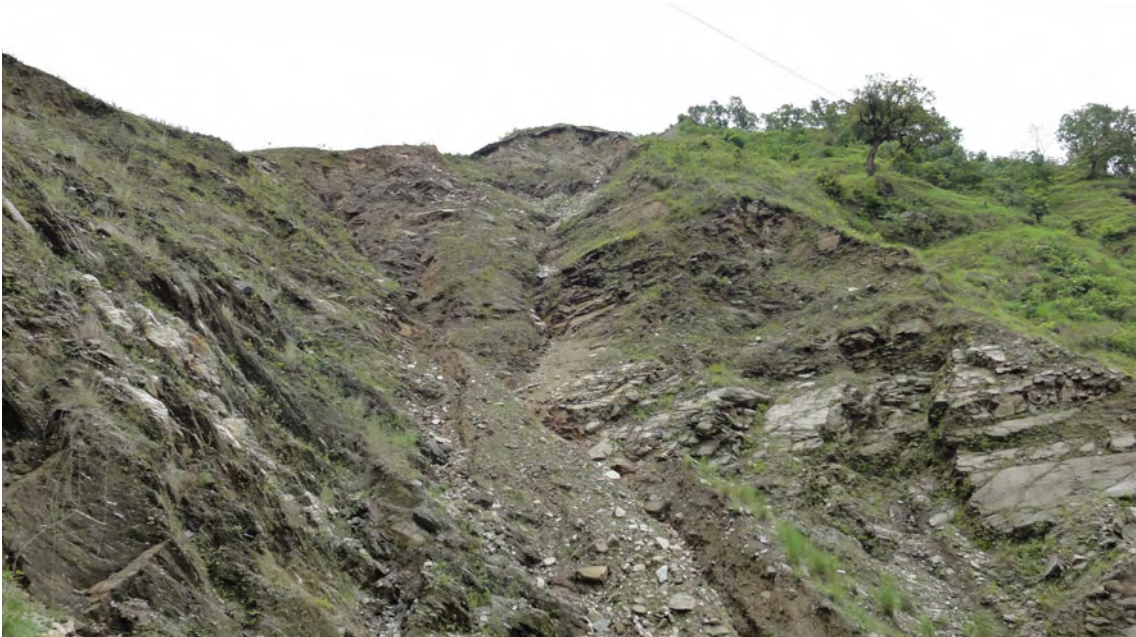
Photo.7 The lower of failure at Sta.18+200.
