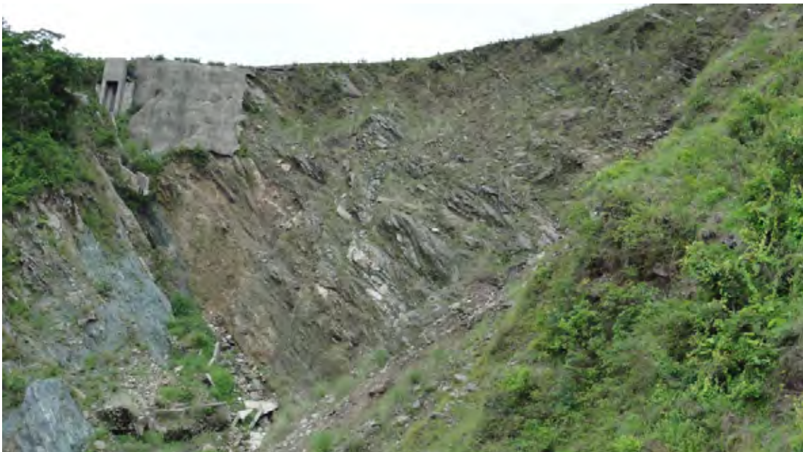
Photo.4 Failure at Sta.17+400.
