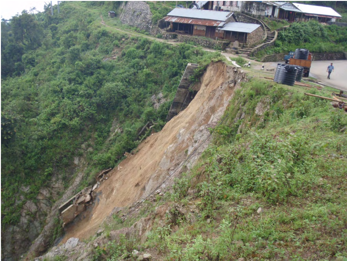
Photo.6 Surface failures at Sta.17+400.
