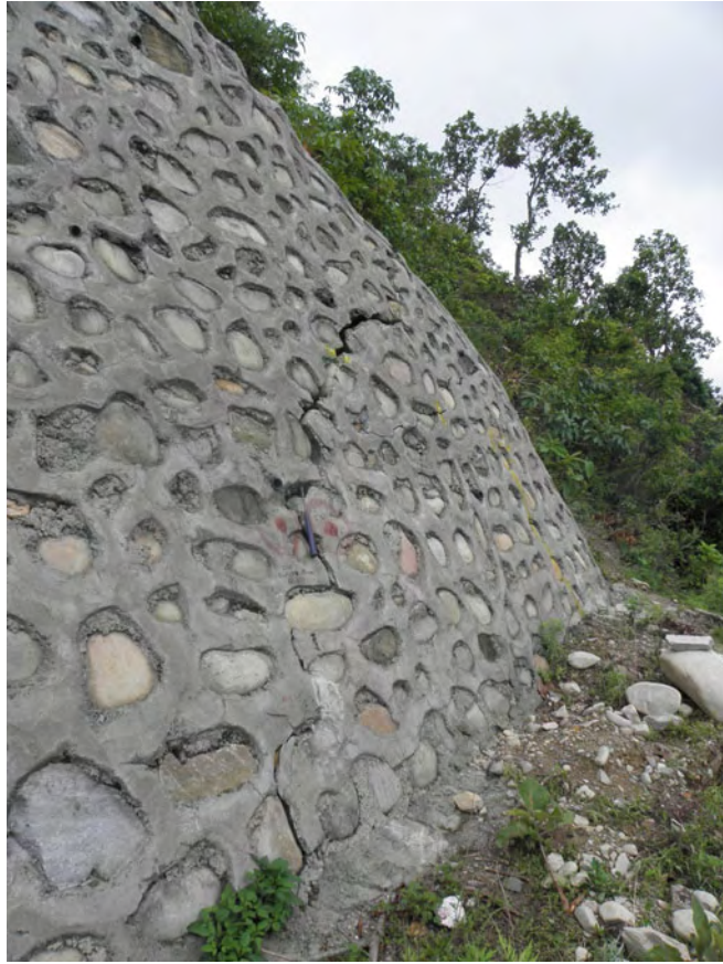
Photo.10 Cracks on the wall at Sta.18+200
