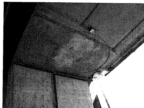
図3.3.3: Rama4橋遊離石灰 (主桁下面)
