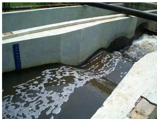
Flow measurement of effluent
