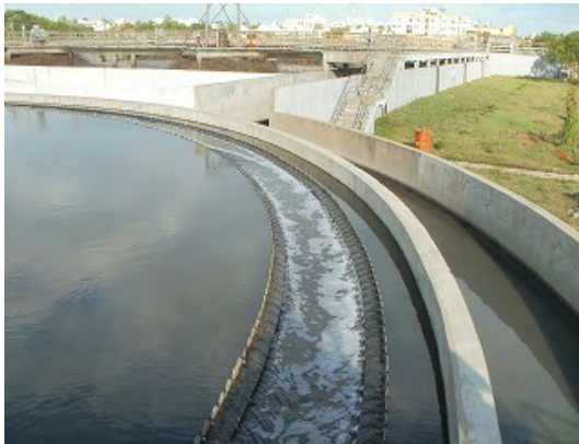
Final sedimentation tank
