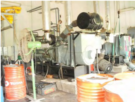
Power generator of digestion gas
