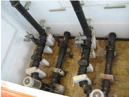
Discharge valve is a electric type
