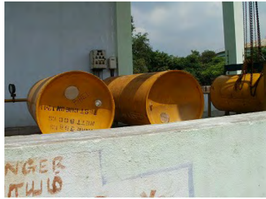
The gas tank of chlorine
