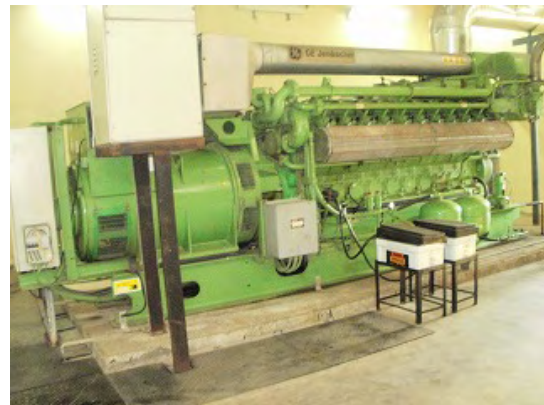
Power generator of digestion gas
