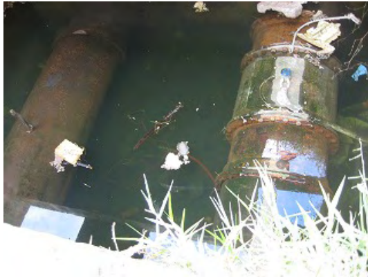
Broken electromagnetic flowmeter
