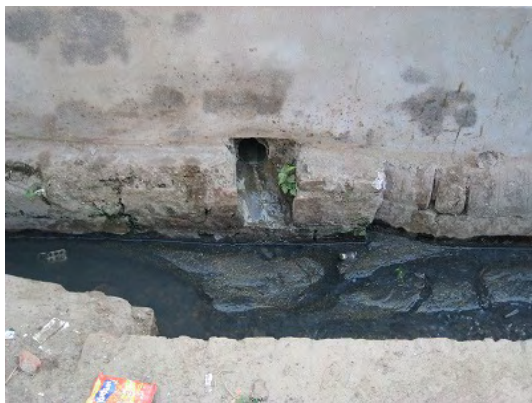
Gray water channel
