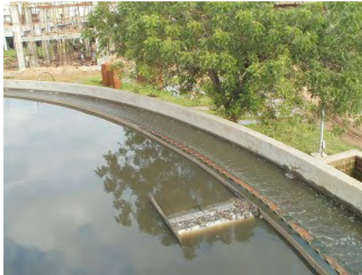
Primary sedimentation tank
