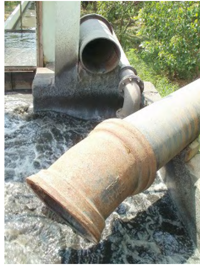
Pipe of recycle flow and excess sludge
