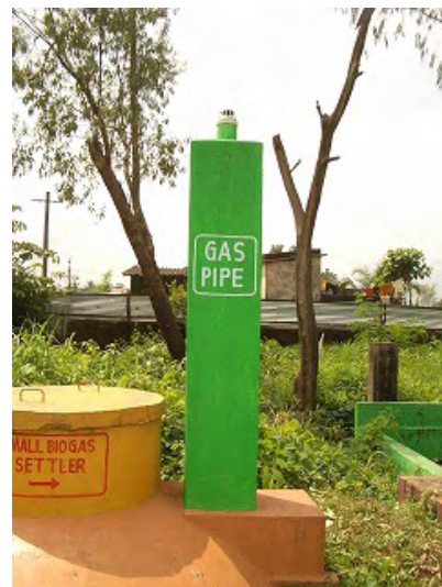
Small Biogas Settler and Gas Pipe
