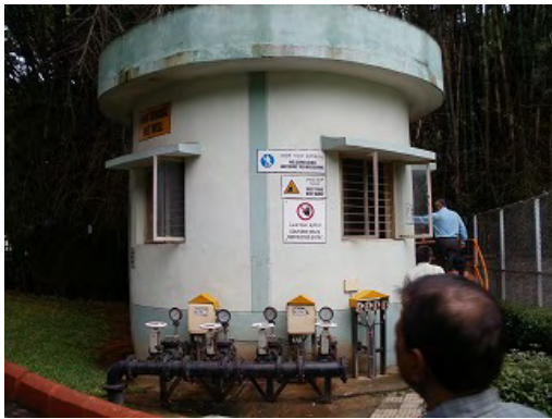
Raw Sewage Wet Well and Pumping
