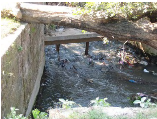
Gray water channel
