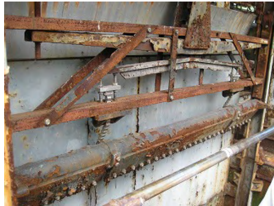
The corrosion of a screen is intense
