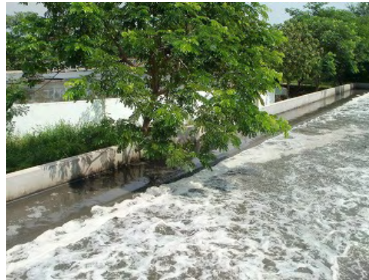
Aeration tank entrance
