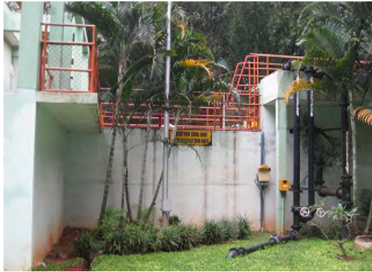
Membrane Bio Reactor
