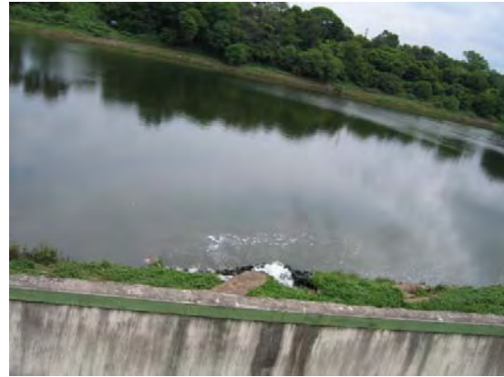
Effluent channel to River
