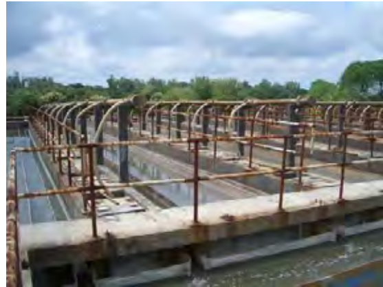
High corrosion in many parts of UASB reactor
