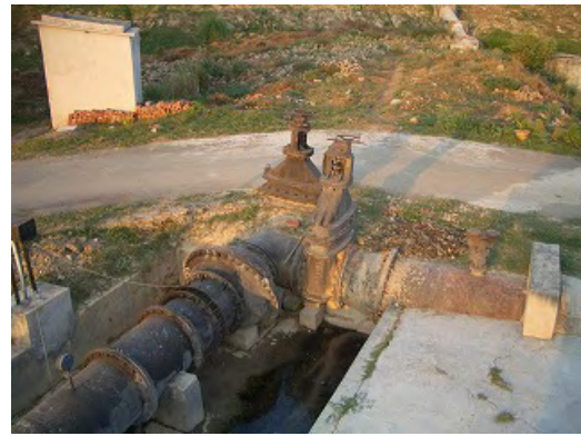
Stormwater by-pass sewer
