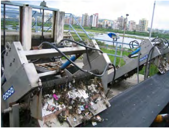
Solid waste from screen passed on to conveyor belt
