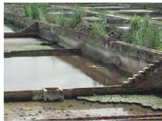
Another view of sludge drying beds
