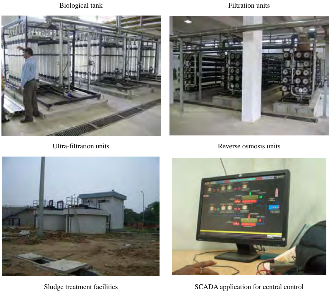
Figure 7 Photographs of STP Facilities at IGIA STP
