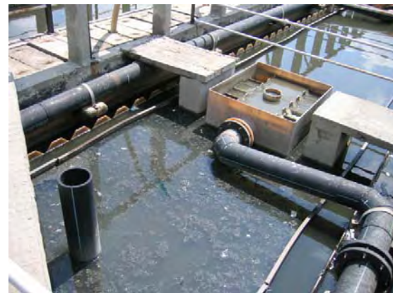
Unequal flow in distribution box of UASB
