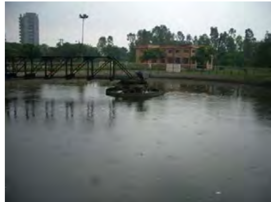
Final settling tank
