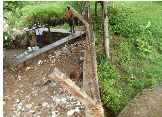
Water flowing into STP from the river (Nala)
