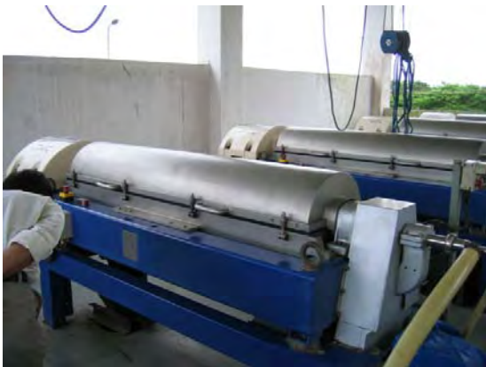
Centrifuge for dewatering of sludge
