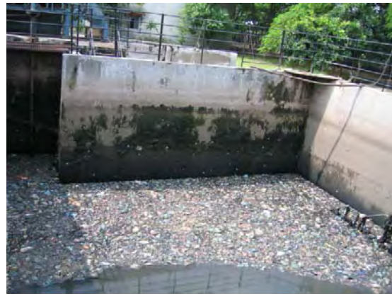
Solid waste in wet well of pumping station
