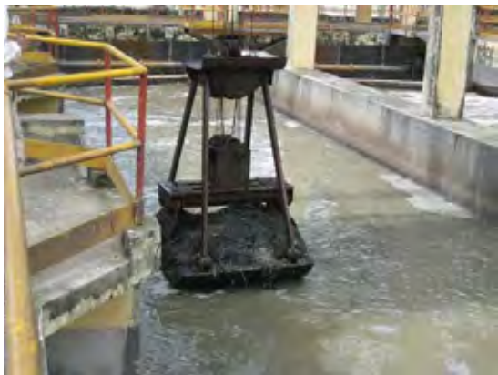
Mechanical grit removal
