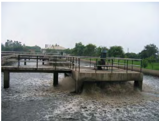
Aerators at STP
