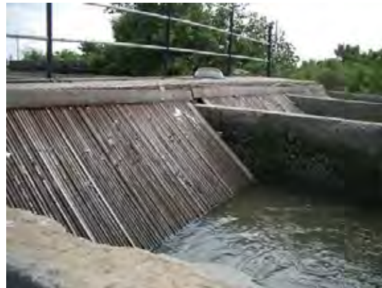
Screen before grit channel
