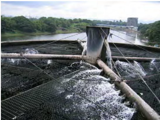
Flow at the top of biotower
