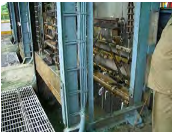
Screen before aerated grit channel
