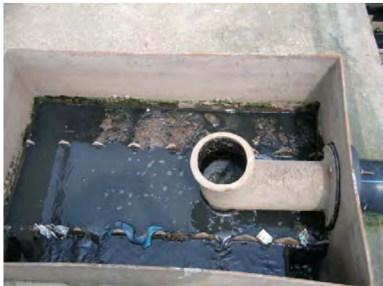
Solid waste reaching even UASB reactor
