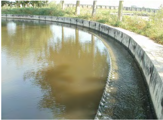
Sludge outflow from final sedimentation tank
