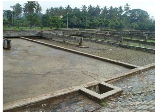
Sludge drying beds
