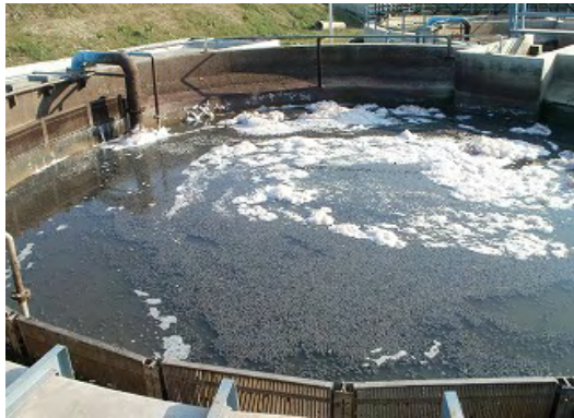
Fluidized Aerated Bed Reactor
