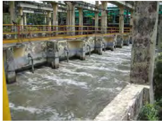
Aerated grit removal tanks
