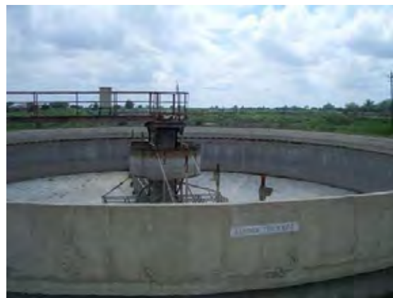
Sludge thickener not in operation
