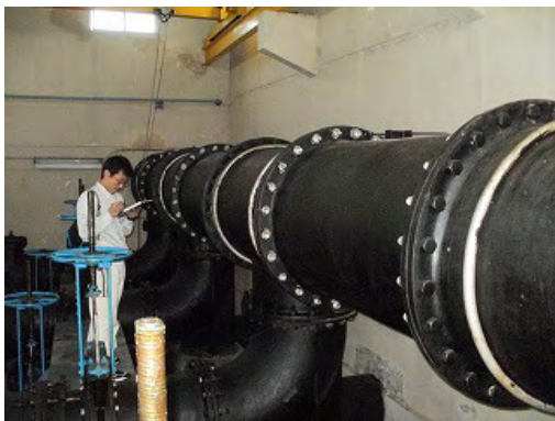
Pipe of return activated sludge
