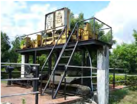
Corrosion in facilities at main pumping station
