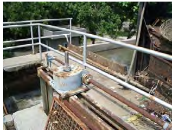
Corrosion in fine screen
