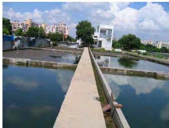
Delayed drying of sludge in drying beds during rainy season
