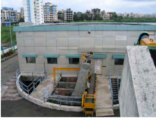
Pumping station conveying water to treatment facilities
