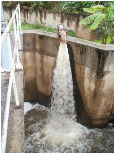
Supernatant flow into wet well
