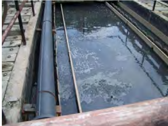
Sludge appearing at surface of UASB reactor
