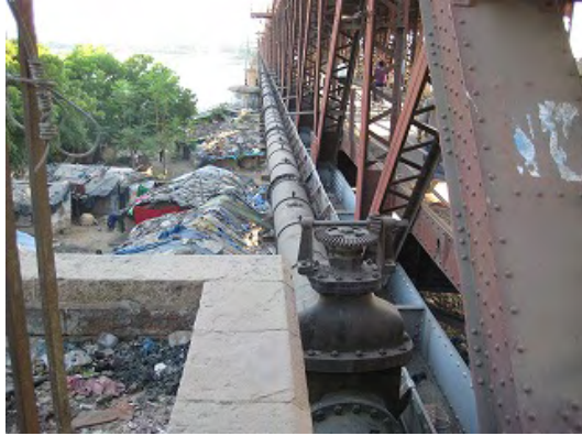
Drain pipe across the Yamuna river
