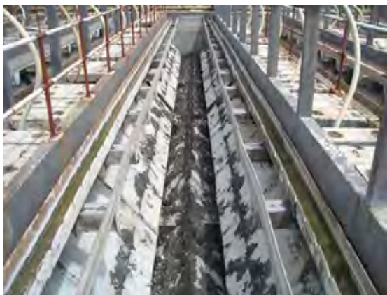
UASB reactor not in operation
