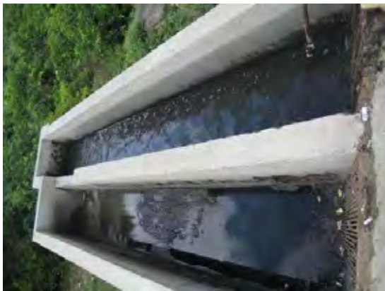
Screen before grit channel
