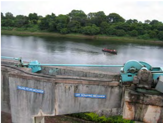
Grit scraping mechanism
