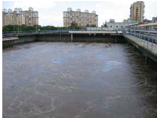
C-Tech Reactor in aeration stage
