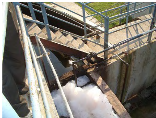
The point of Chlorination
