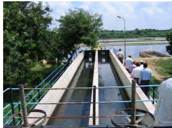
Grit channel and anaerobic pond
