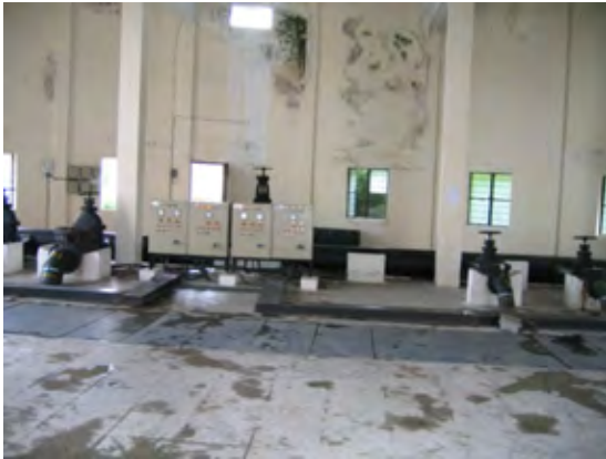
Pumps for pumping influent
