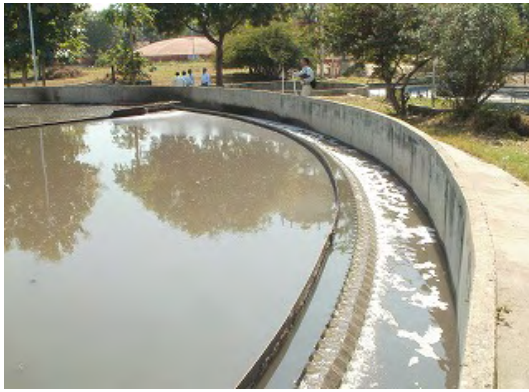
Primary sedimentation tank
