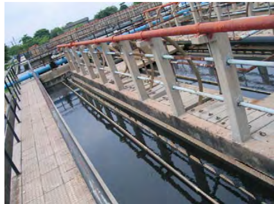
Effluent trough in UASB reactor not in level
