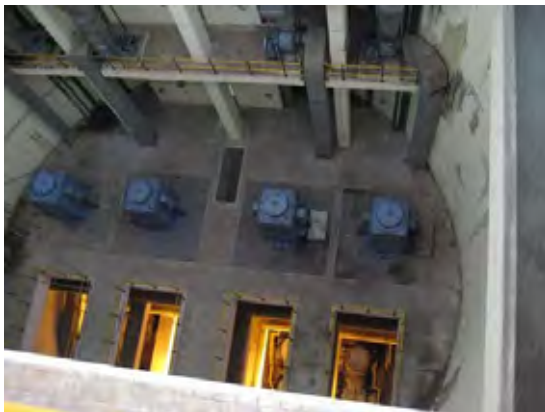
Influent pump view from top
