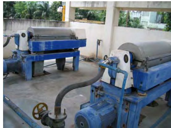
Centrifuge for dewatering
