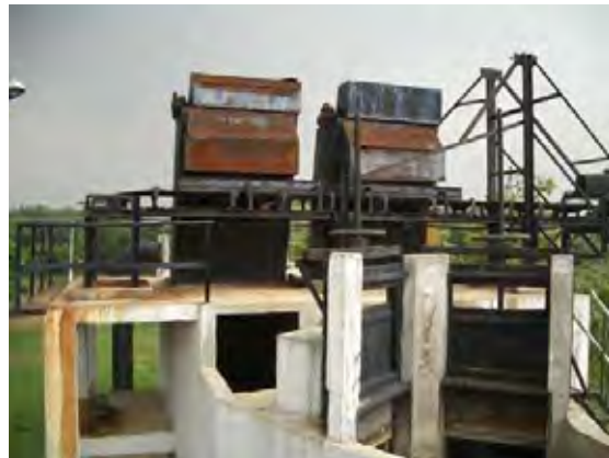
Corrosion in screen
