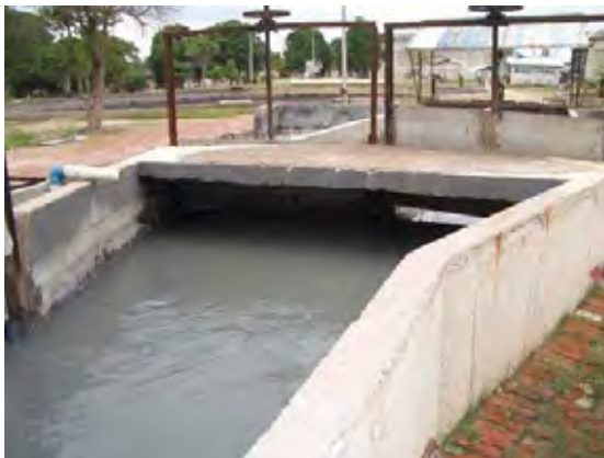
Inlet at STP
