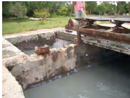
Screen before grit channel
