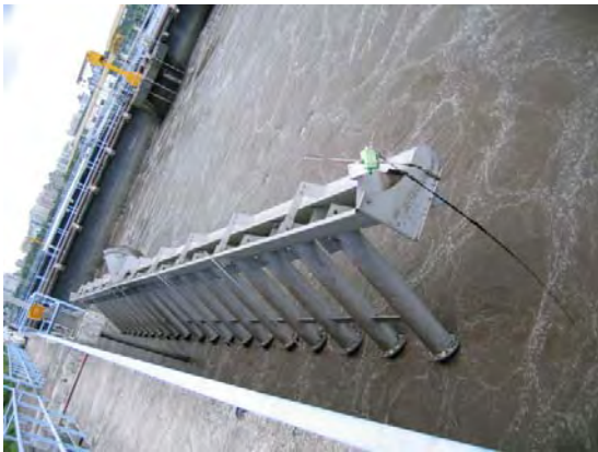
C-Tech Reactor in filling and aeration stage
