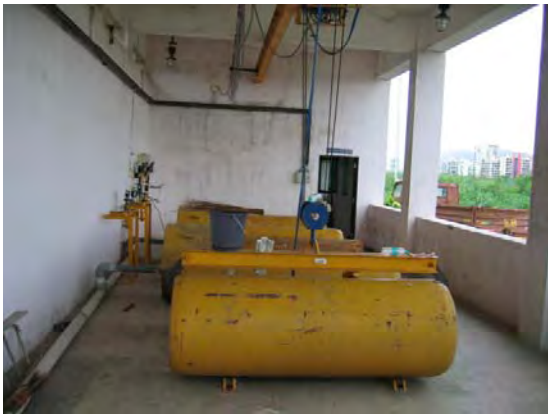
Cylinder for chlorination
