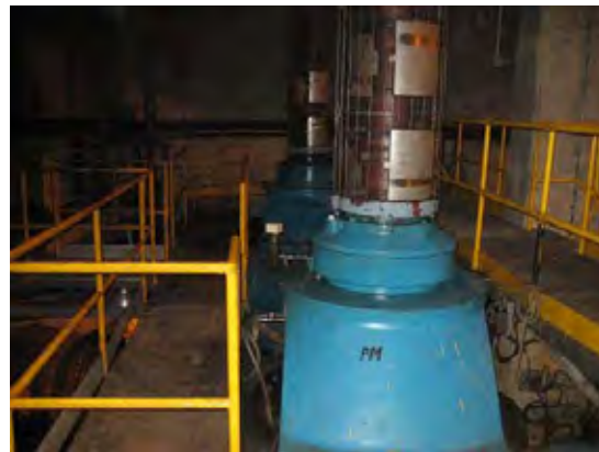
Large capacity influent pump
