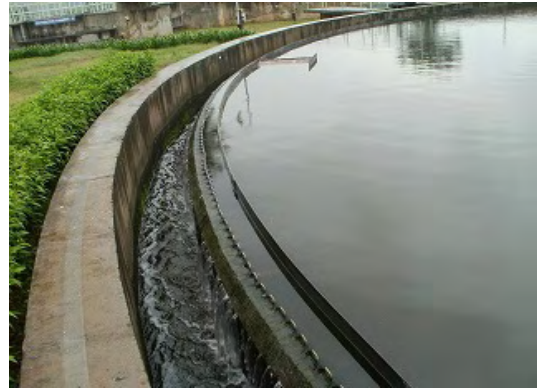
Final sedimentation tank
