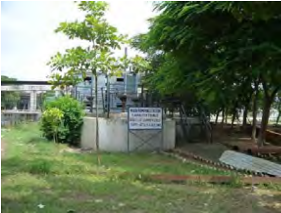
Main pumping station in STP premises
