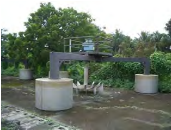
View of aerator used in lagoon
