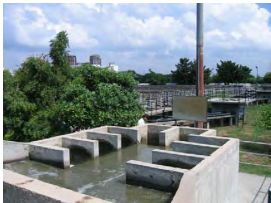
Distribution chamber to UASB reactor
