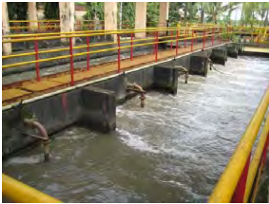
Aerated grit channel
