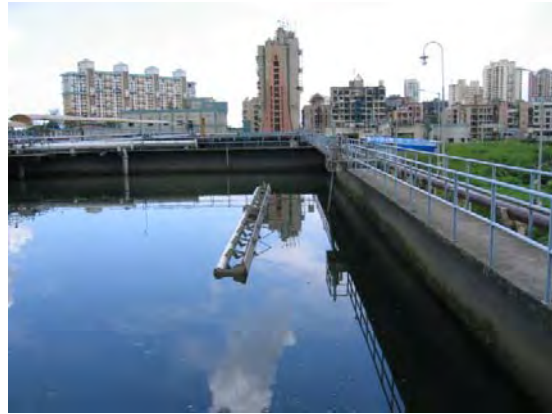
C-Tech Reactor in decantation stage
