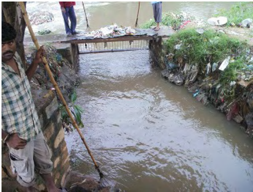
Water flowing into STP from the river (Nala)
