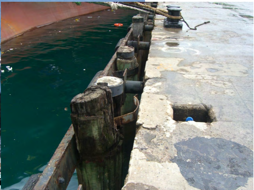
Deteriorated to a substantial extent
