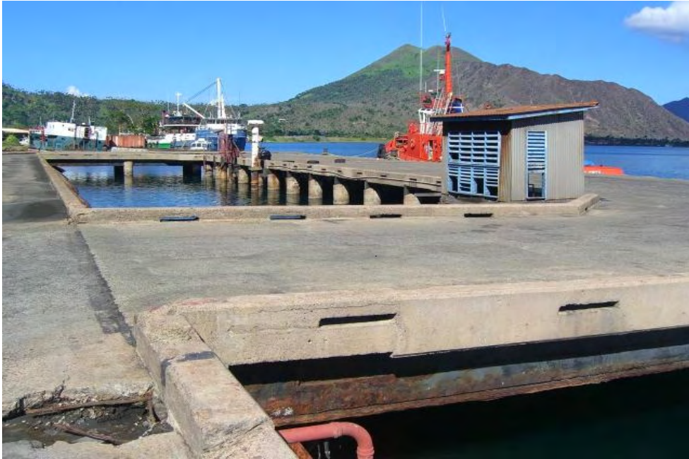
Photograph 6.5 The State of Berth 1
