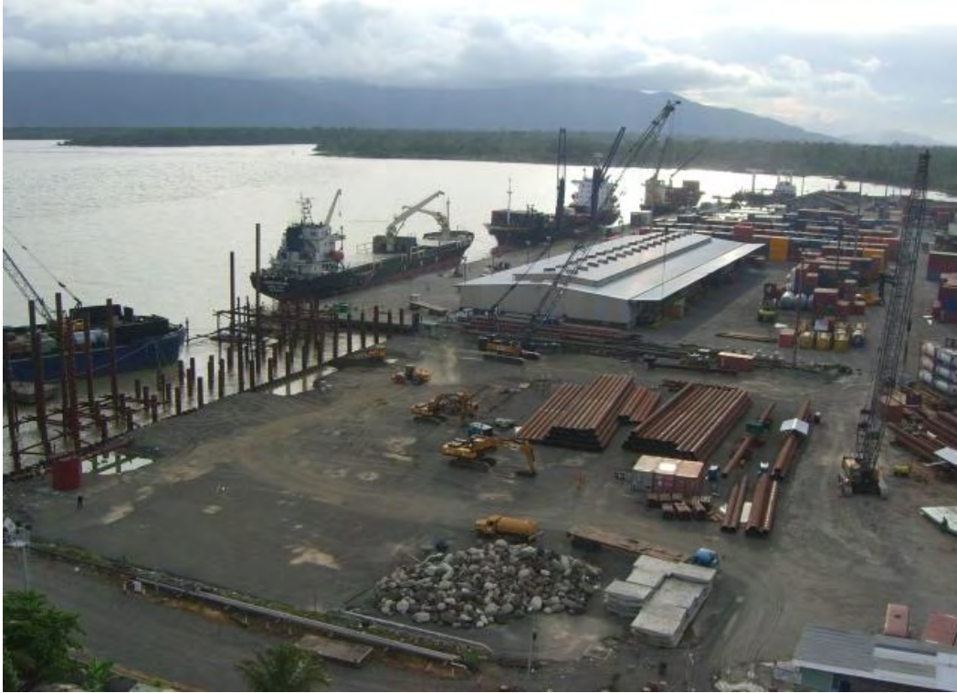
Photograph 6.3 The Current State of Lae Port (area in the foreground is where construction is currently underway)
