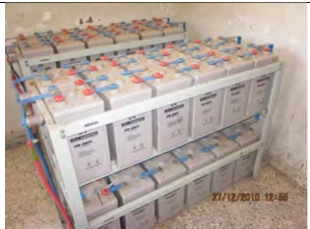
ZTE Local Exchange Batteries
