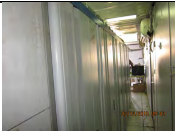
ZTE Exchange Rack
