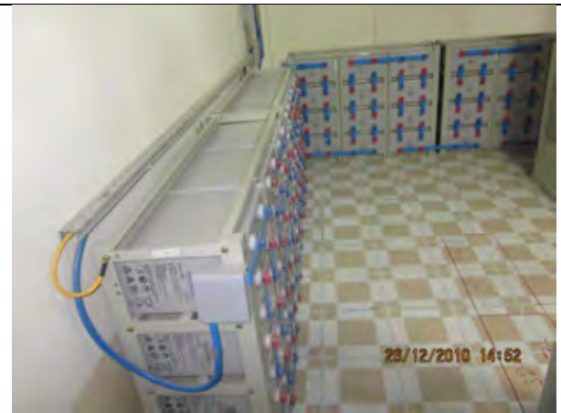
Optical Project Batteries
