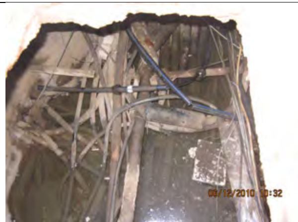
Cables inside Man Hole
