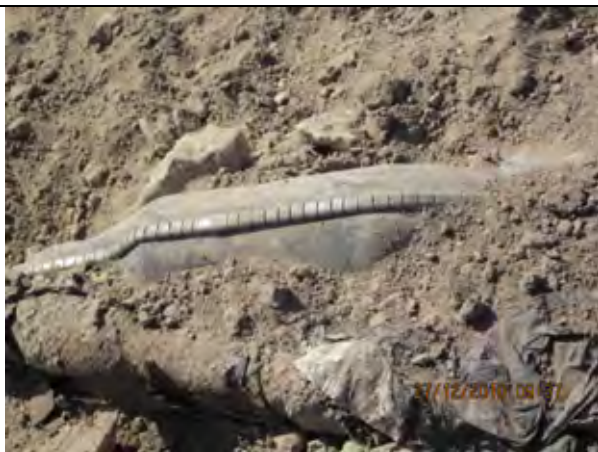
Cable Joint on the Street
