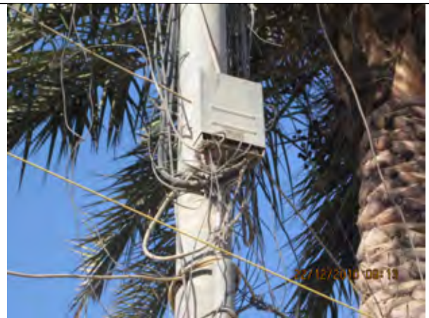
Telephone Distribution Box
