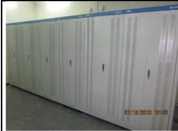
ZTE Local Exchange Rack
