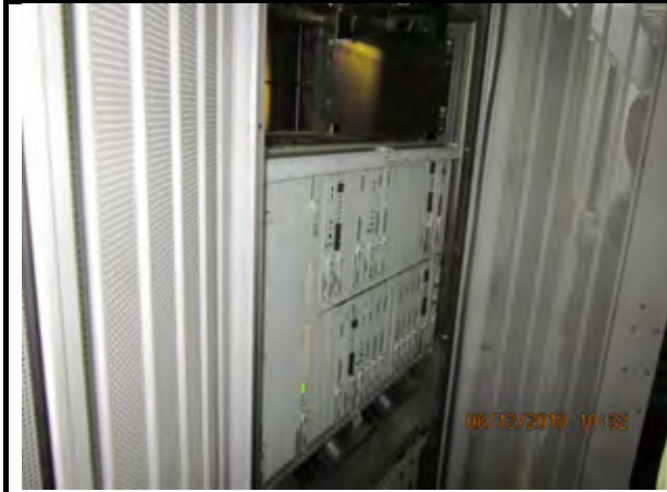
Exchange Control Rack
