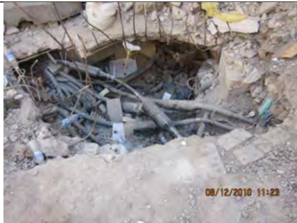
Telephone Cables along the Street
