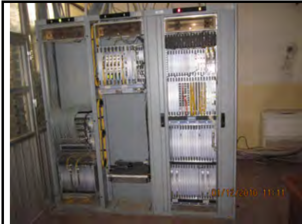
DWDM Transmission Rack
