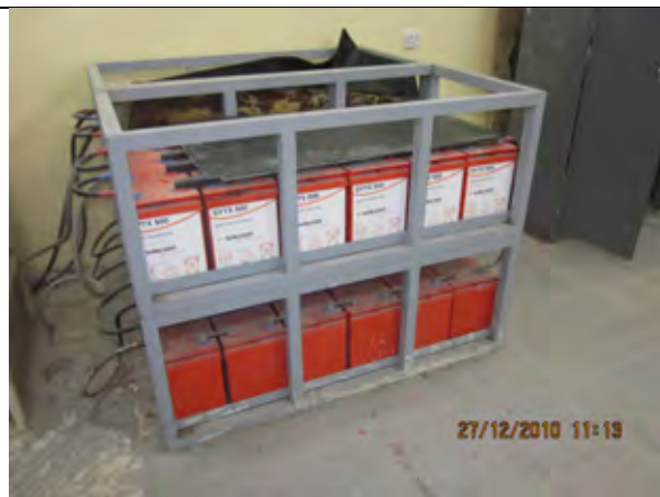
ZTE Local Exchange Batteries
