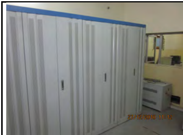
ZTE Local Exchange Rack ( 10,000 lines)
