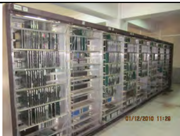
Local Exchange Rack
