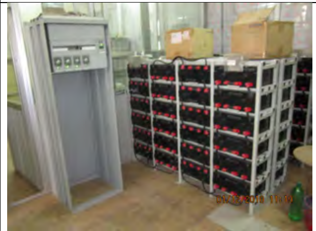
DWDM Rectifier and Battery
