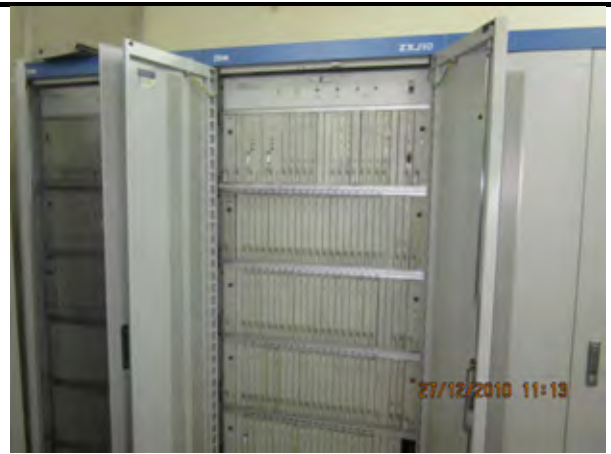
ZTE Local Exchange Rack
