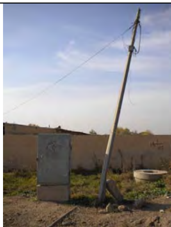
Leaned Telephone Pole
