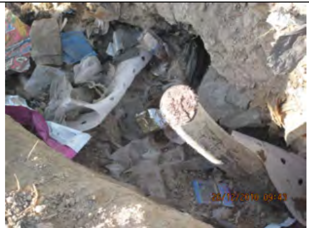
Cable cut along a Street
