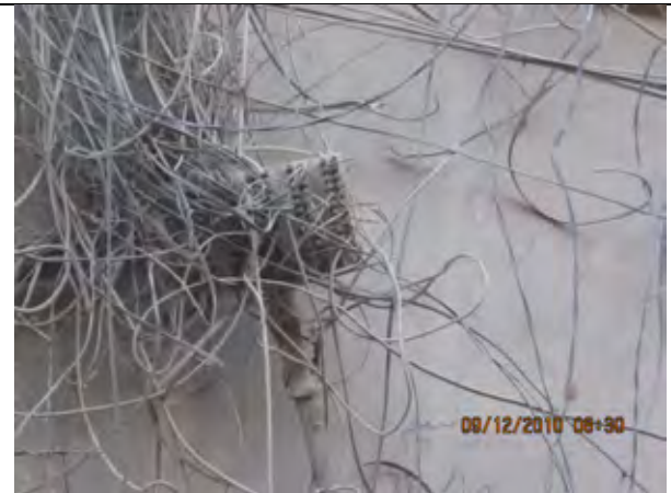
Telephone Distribution Box
