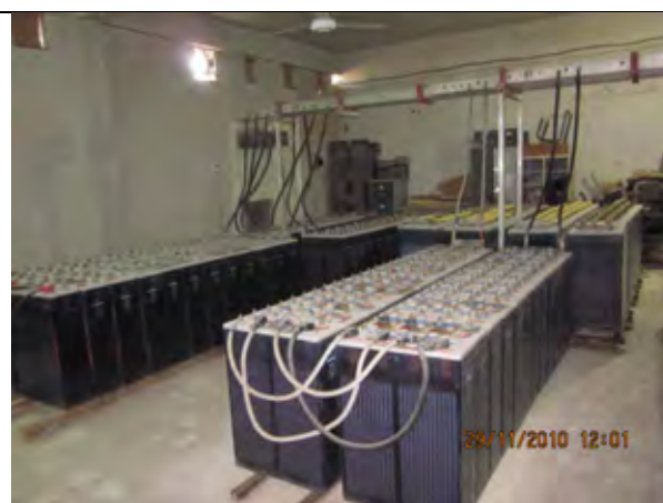
Alcatel Exchange Battery
