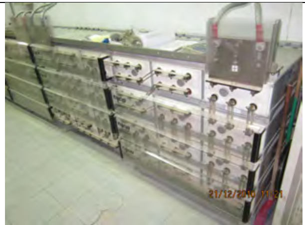
Lucent Local Exchange Batteries
