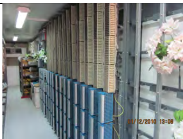
Alcatel Local Exchange DDF
