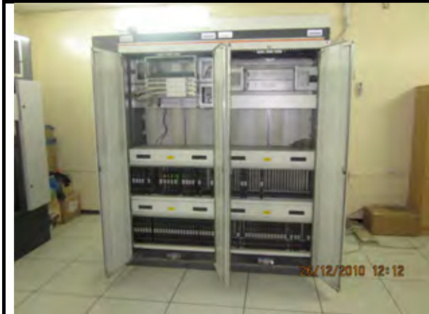
Alcatel Transit Exchange Rack
