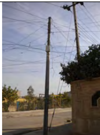
Telephone Pole with Distribution Box
