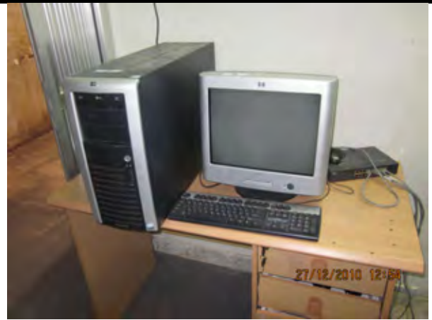
ZTE Local Exchange Work station
