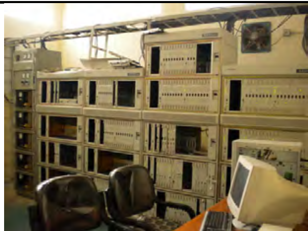
Local Exchange Rack
