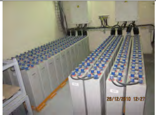
Alcatel Local Exchange Batteries
