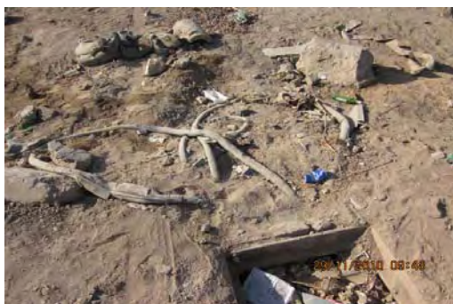
Telephone cables in Baghdad
