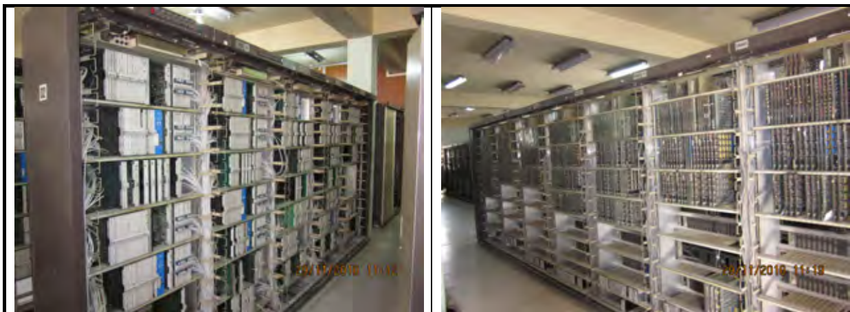
Exchange Signaling Rack
