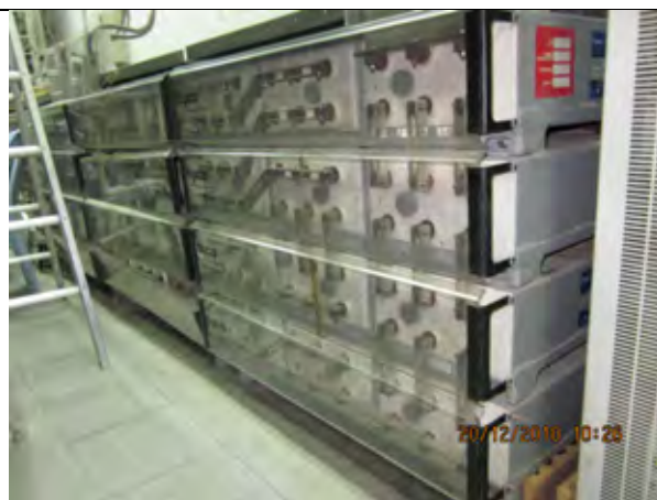
Lucent Exchange Batteries
