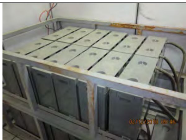
ZTE Exchange Batteries
