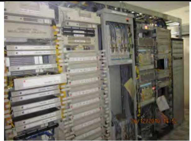
Optical Project Rack
