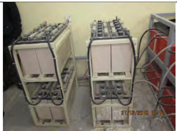
ZTE Local Exchange Batteries
