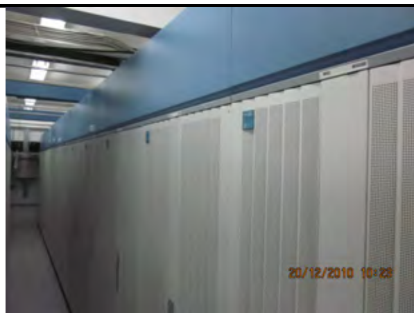
Lucent Local Exchange Rack
