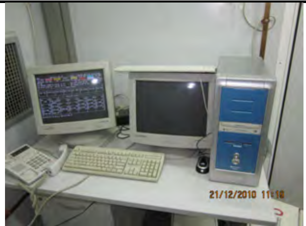
Lucent Local Exchange Work station
