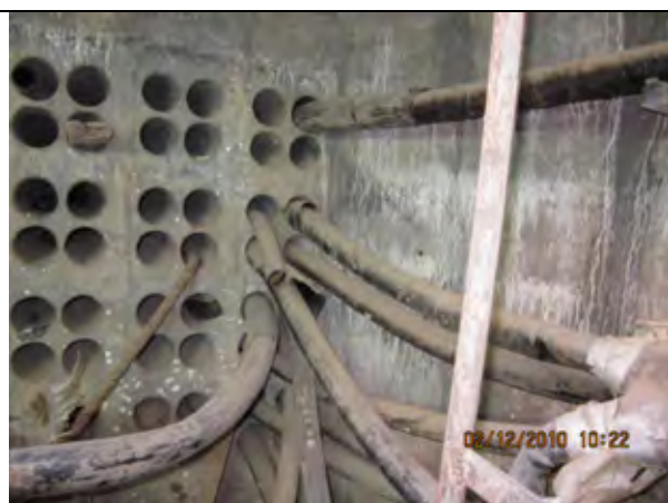
Cables inside Manhole
