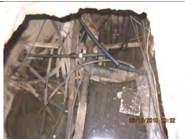
Cables inside Man Hole
