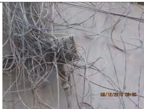
Telephone Distribution Box
