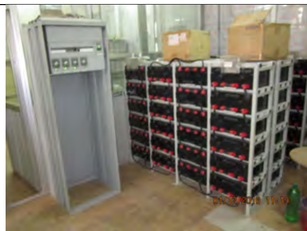
DWDM Rectifier and Battery
