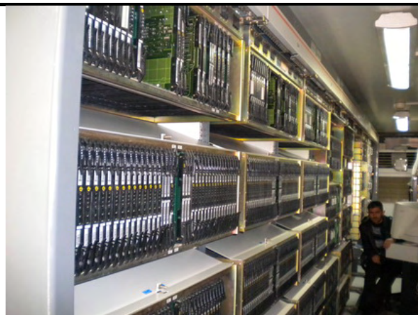
Alcatel Exchange Rack
