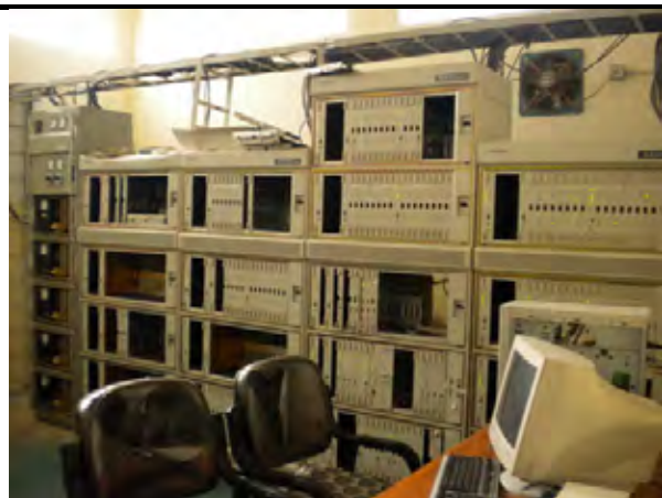
Local Exchange Rack
