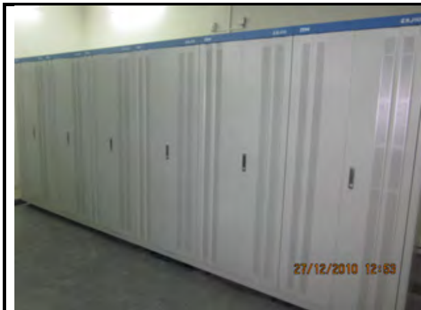
ZTE Local Exchange Rack
