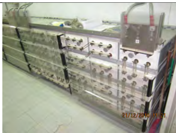
Lucent Local Exchange Batteries
