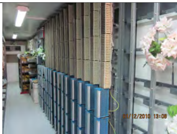
Alcatel Local Exchange DDF
