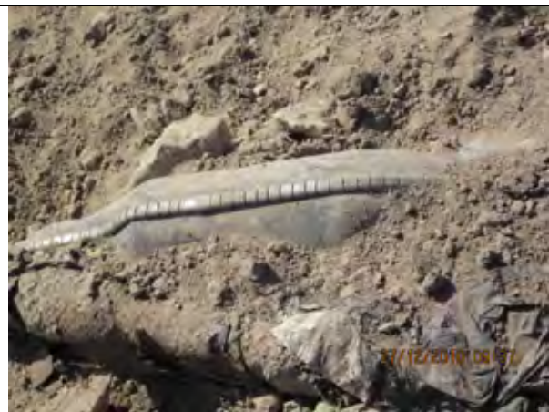
Cable Joint on the Street
