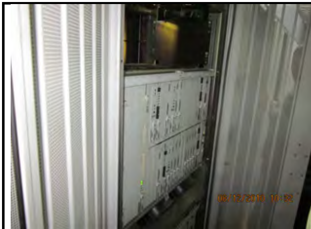
Exchange Control Rack
