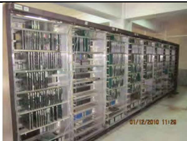
Local Exchange Rack
