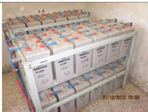
ZTE Local Exchange Batteries
