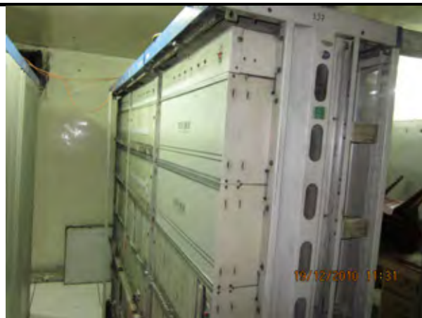
ZTE Local Exchange Rack
