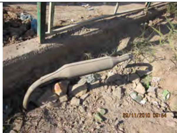
Cable Joint in the Street
