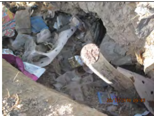
Cable cut along a Street
