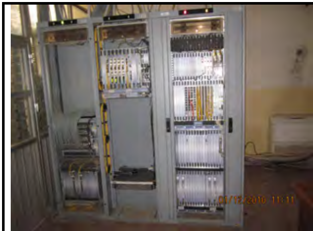
DWDM Transmission Rack
