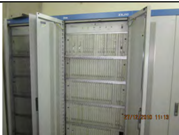
ZTE Local Exchange Rack
