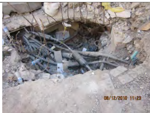
Telephone Cables along the Street
