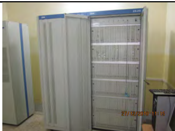
ZTE local Exchange Rack (3,000 lines)
