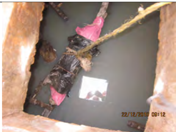
Cable Closure inside Man Hole filled with Water
