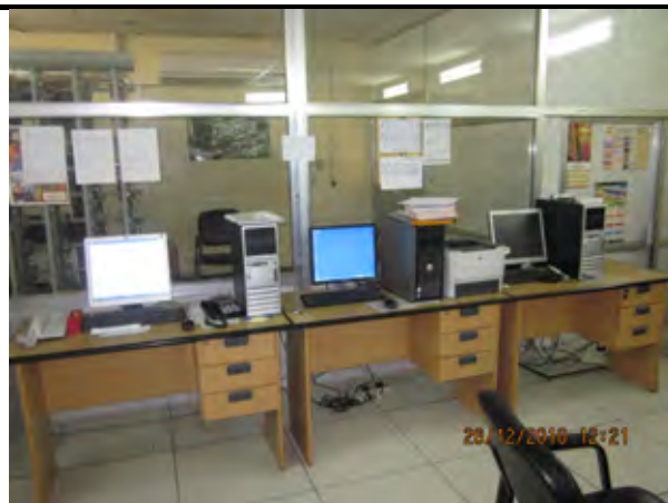
Alcatel Transit Exchange Work Station
