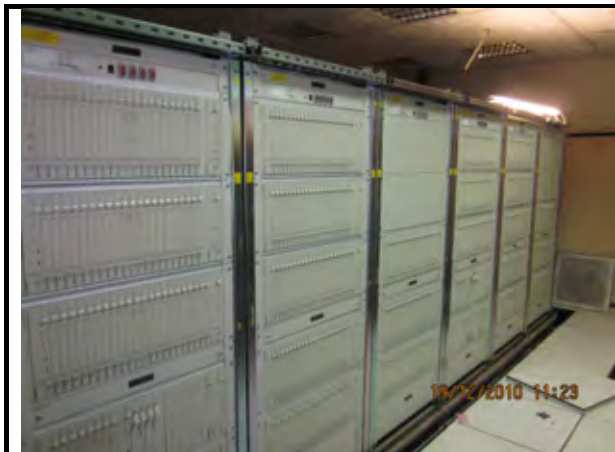
Quicktel Local Exchange Rack
