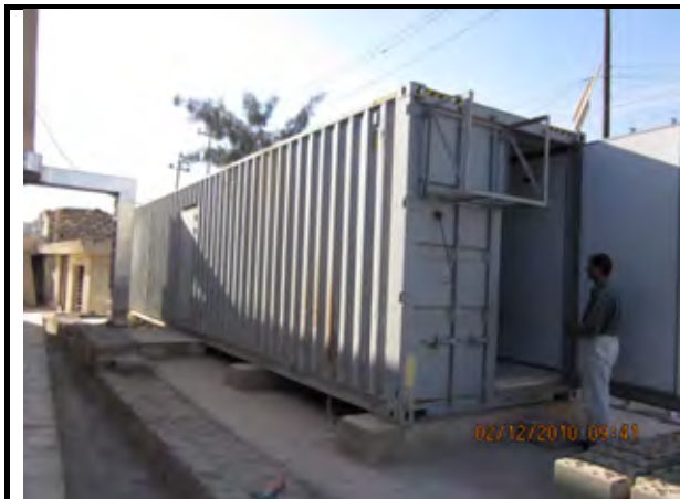
ZTE Exchange Container
