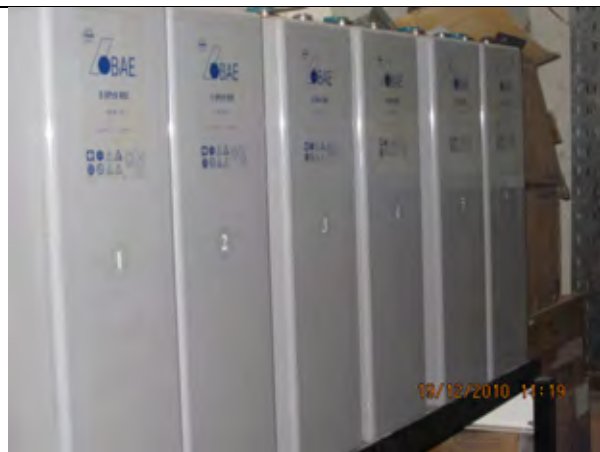
Quictel Transit Exchange Batteries
