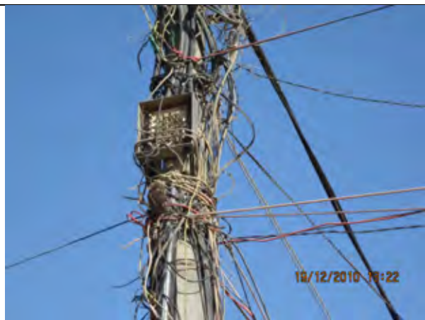
Telephone Distribution Box
