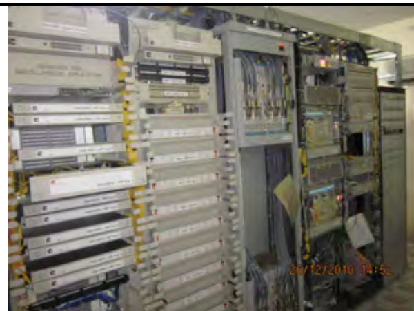
Optical Project Rack
