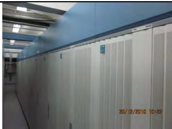
Lucent Local Exchange Rack
