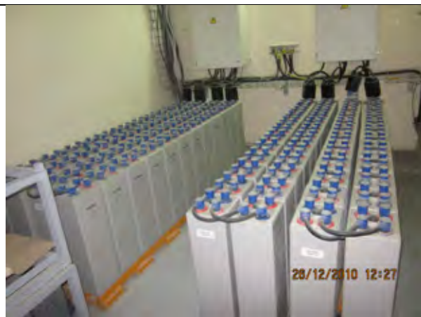
Alcatel Local Exchange Batteries
