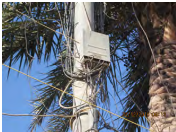
Telephone Distribution Box
