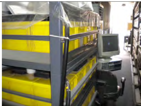
Alcatel Exchange Batteries
