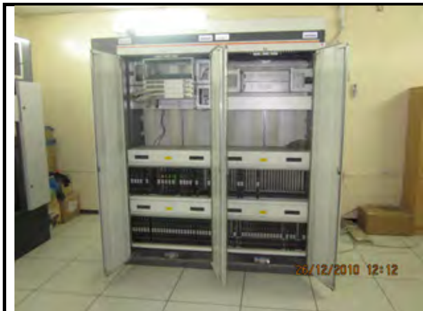
Alcatel Transit Exchange Rack
