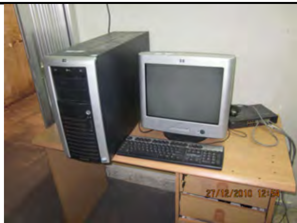
ZTE Local Exchange Work station
