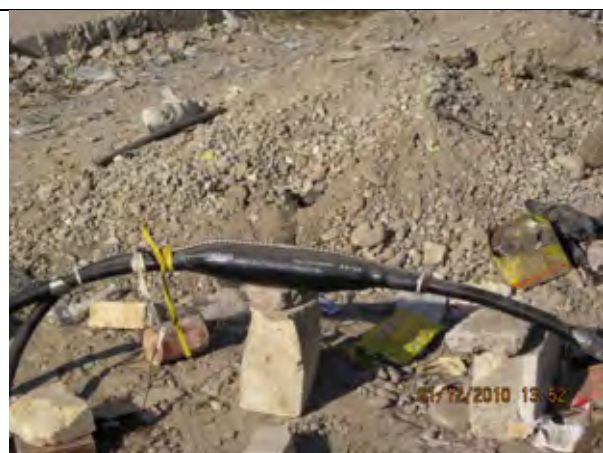
Cable Joint in the Street
