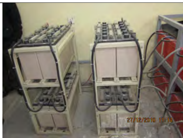
ZTE Local Exchange Batteries
