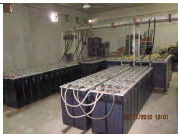
Alcatel Exchange Battery
