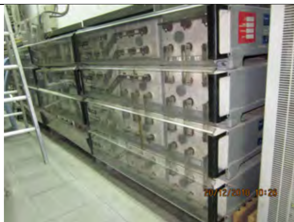
Lucent Exchange Batteries
