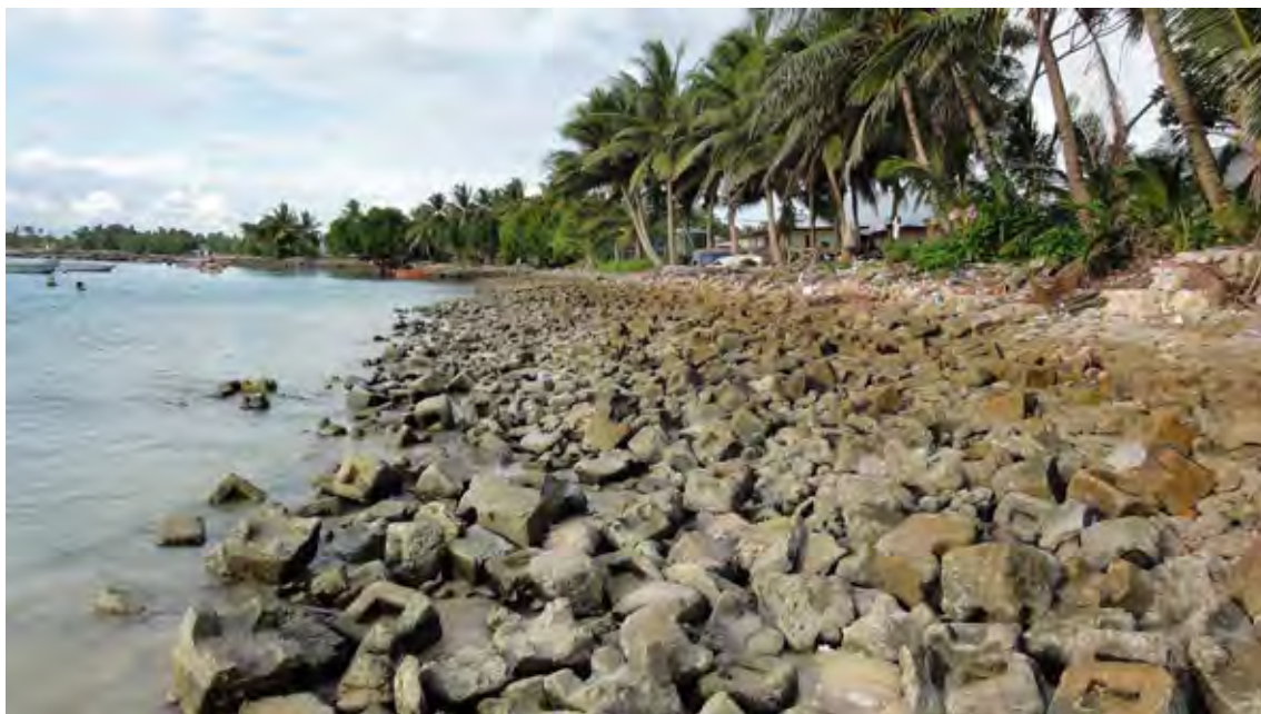
Photo 11.1 Collapsed Seawall (Unconsolidated Cube-type Blocks)
