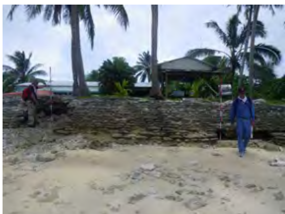
Photo 5.28 A Privately-Implemented Seawall – a Wet Masonry Seawall to the North of Vaiaku Lagi Hotel (partially collapsed)
