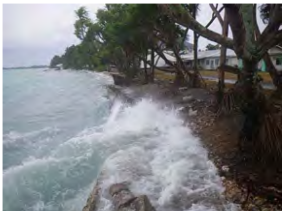
Photo 5.26 Wave Run-ups in front of a Vertical Seawall - the Mixed Vertical/Sloping Seawall in front of Vaiaku Lagi Hotel
