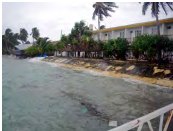
Photo 5.27 Wave Run-ups in front of a Vertical Seawall – A vertical Seawall on the Northern Side of Vaiaku Wharf
