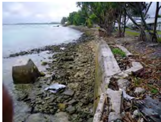
Photo 5.25 A seawall Implemented as a Public Work – a Vertical Seawall on the Northern Side of Vaiaku Wharf (Remnant of part of a gabion seawall is seen.)
