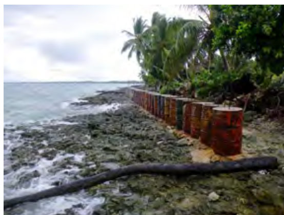
Photo 5.29 A Privately-Implemented Seawall – a Seawall at the Coastal Area at the Southern End of Funafuti Constructed with Concrete-Filled Oil Drums
