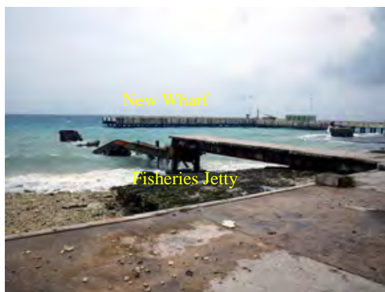
Photo 5.2 Collapsed Fisheries Jetty
