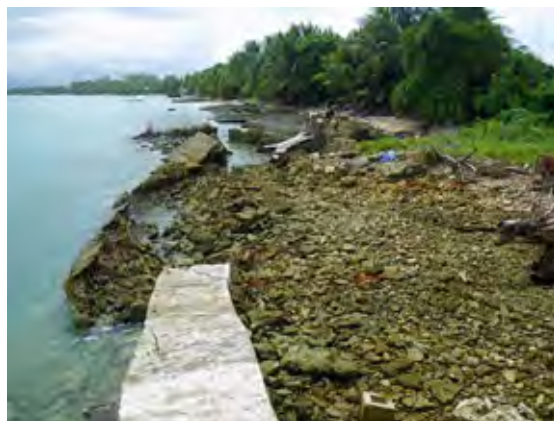
Photo 5.31 A Privately-Implemented Seawall – Collapsed because of Inappropriate Structure
